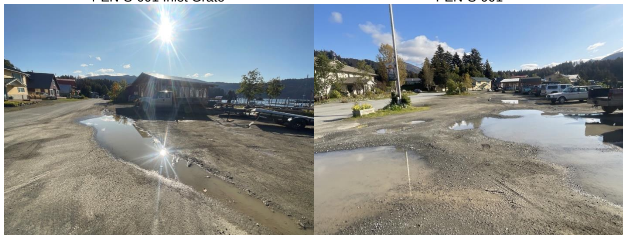
Ponding in Front of Gateway Pavilion
