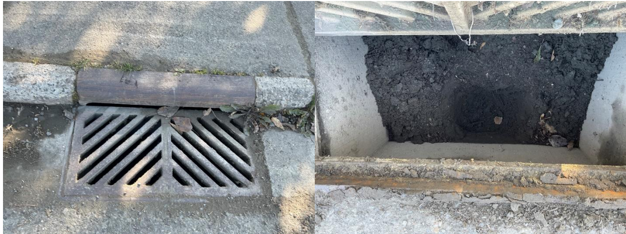
PEN-S-001 Inlet Grate
