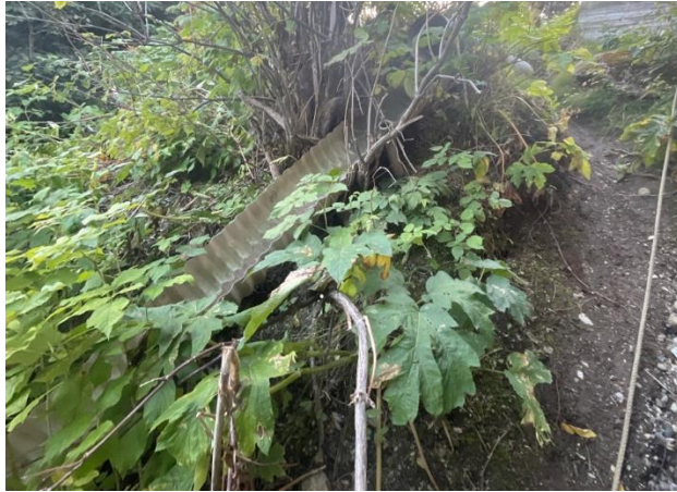
ARIP-S-003 Outlet and ARP-P-003 Flume
