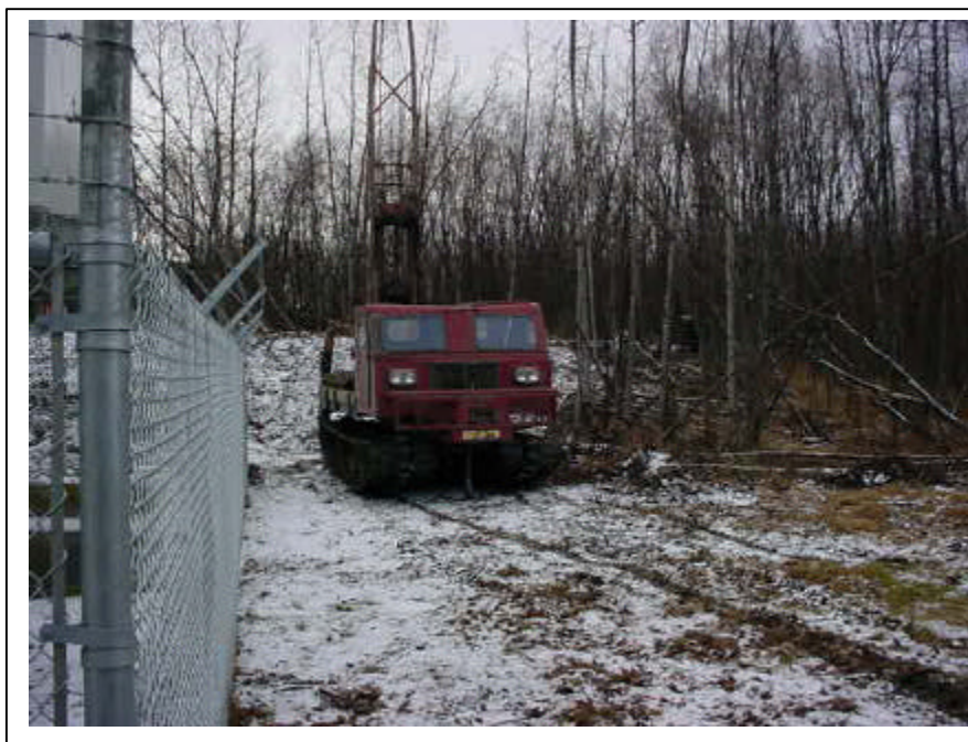
Photograph 14: Looking southwest, Boring B3 was advanced adjacent to the southwest corner of the fuel tank storage fence.
