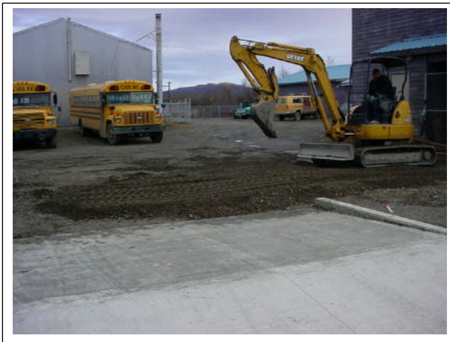
Photograph 9: Looking northeast, the southeast septic trench was compacted with the tracks of the backhoe following backfill activities.
