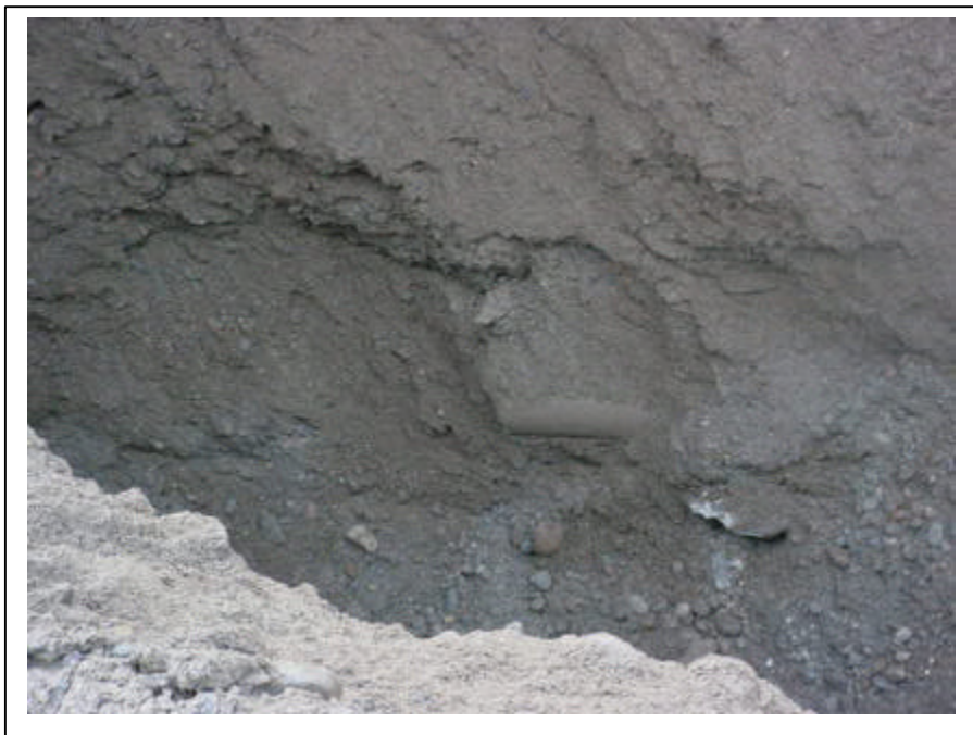
Photograph 5: Looking down into the southeast end of the southeast septic trench, a break was observed in the former septic line.
