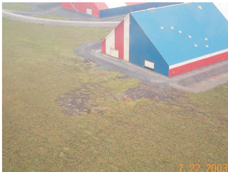
Photograph 49. Aerial view of stressed vegetation to the northwest of CSB1.
