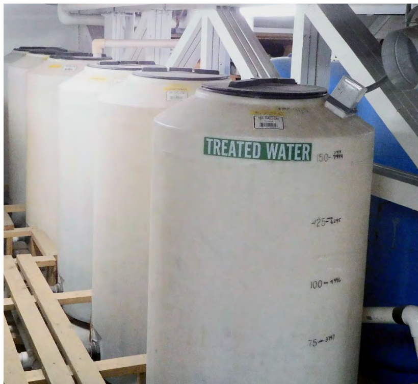
Exhibit 5-2: Current Treated Water Storage
