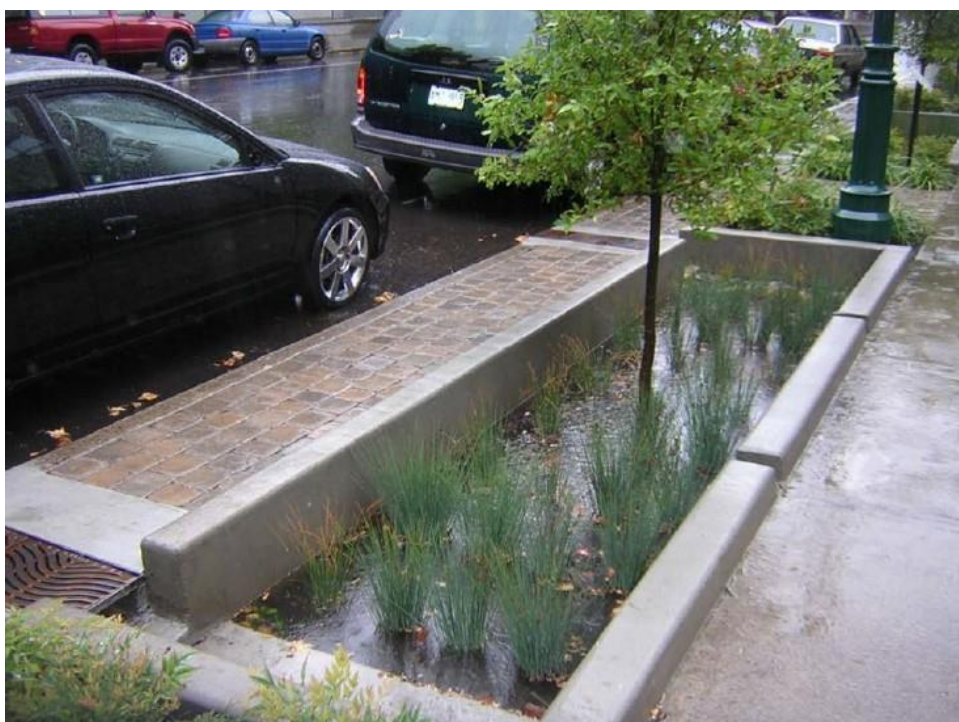
Figure 18. Trench drains (covered with iron grates) in a pedestrian strip convey stormwater from curb and gutter to a bioretention planter.
