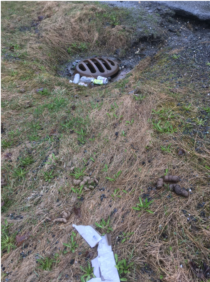
Figure 12. Pet waste near a catch basin in the Crest Street right-of-way. An example of a bacteria source in the Lower Jordan Creek watershed. (SAWC photo)
