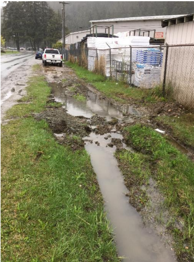
Figure 33. Vehicles parked in a swale in the Crest Street right-of-way near Valley Lumber. View looking north near the east end of Mallard Street in March 2020.
