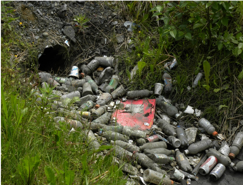
Figure 13. Litter in a drainage ditch along Trout Street in the Lower Jordan Creek Watershed.
