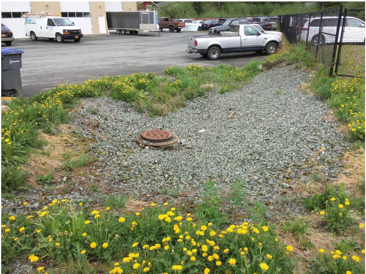
A stormwater infiltration basin at the north end of Jordan Ave. is designed to receive runoff from a parking lot near Jordan Creek.
