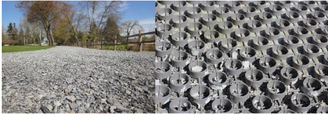
Figure 5. Left: park access road constructed with plastic grid and gravel. Right: plastic grid system (Washington Stormwater Center LID Training Manual).
