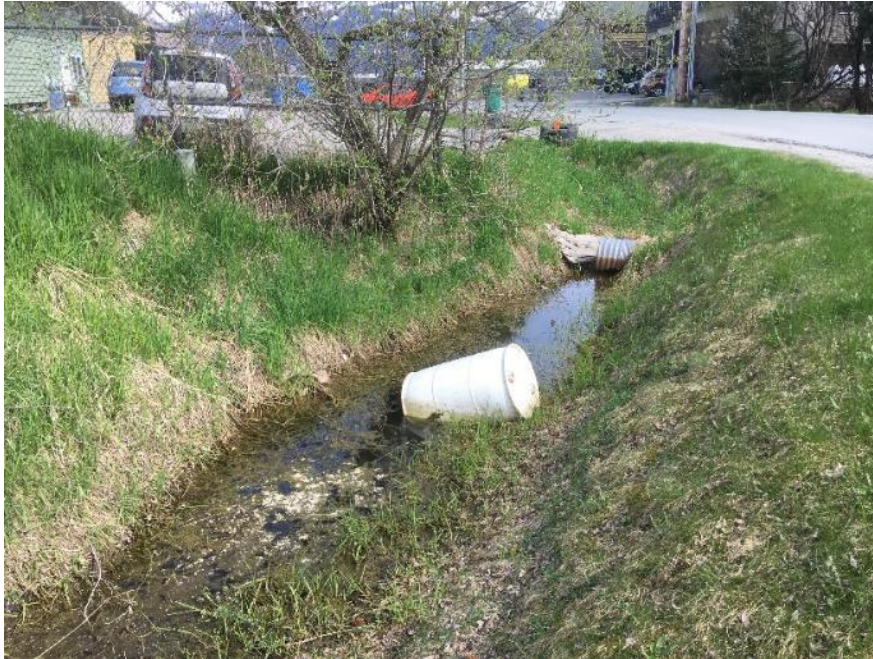
Figure 57. Stormwater runoff pools in a ditch at the junction of Alpine Ave. and Airport Blvd. View looking southeast in May 2020.
