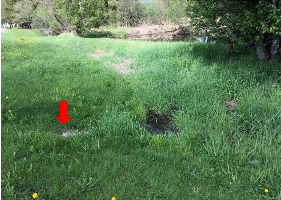
Figure 53. The Yandukin Drive East stormwater system discharges runoff from a pipe (indicated by red arrow) into a grass swale next to Jordan Creek. Jordan Creek is visible at top of photo. View looking northwest from the north side of Yandukin Drive in May 2020.
