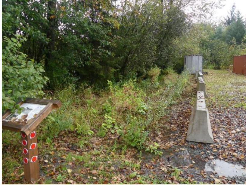
Figure 8. An infiltration trench (left of barriers) on the west side of Jordan Creek, downstream of Glacier Highway in Juneau. Runoff enters from the lower right of photo; Jordan Creek is left of photo.
