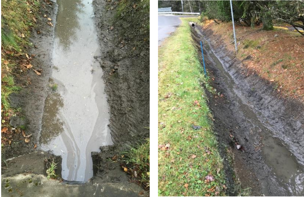
Figure 10. Left: Oil residue on stormwater runoff in the Trout Street Ditch. Right: The Trout Street Ditch following maintenance to remove vegetation and sediment. View looking northwest towards Jordan Creek in October 2018.
