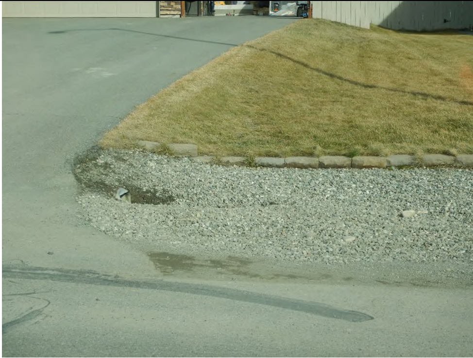
Crushed driveway culvert along Fetlock Drive.
