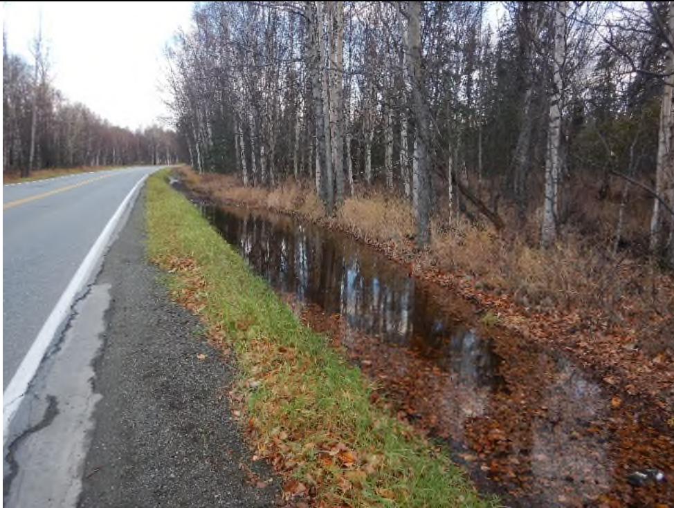
Ponding in ditches/ATV trails along Stringfield Road.
