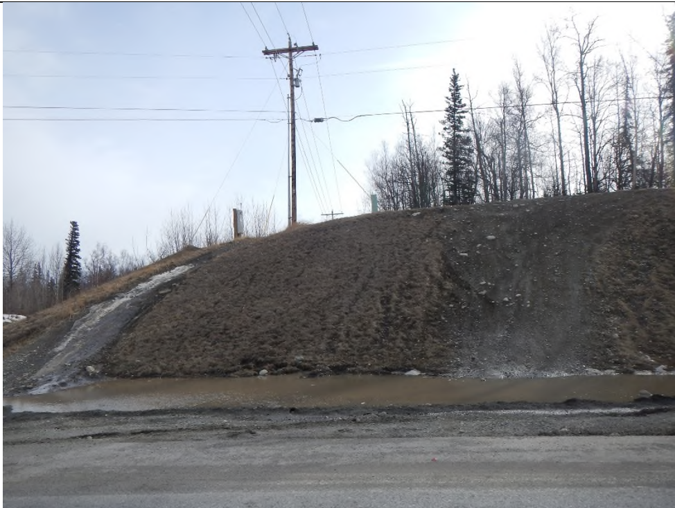
Ponding along Trunk Road.
