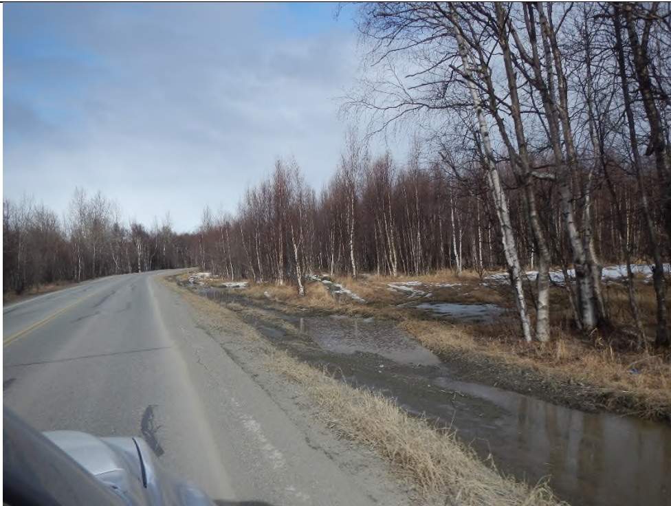
Ponding in ditches/ATV trails along Stringfield Road.
