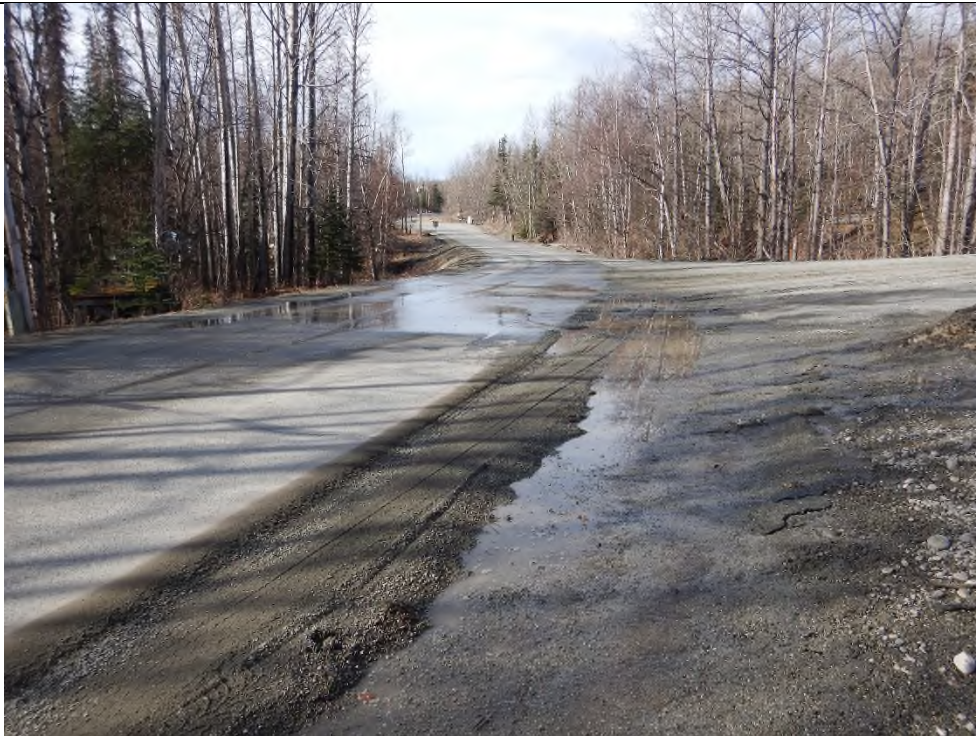
Roadway ponding at Wilderness Drive.
