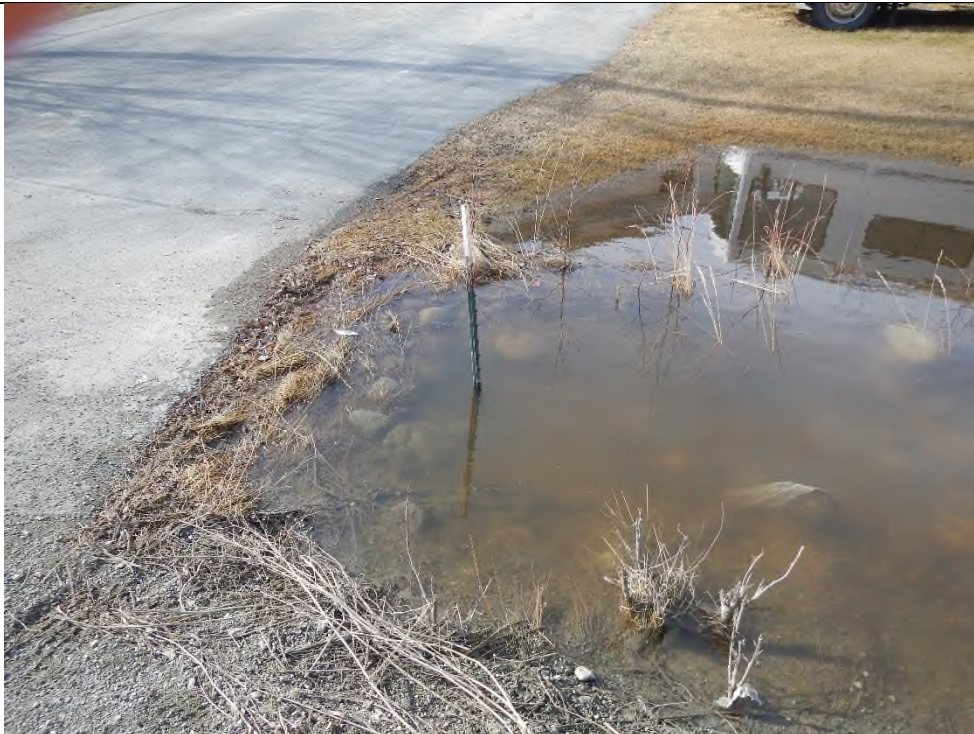
Blocked driveway culvert at Vickie Circle.
