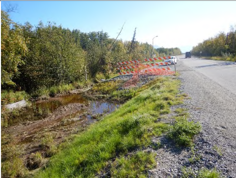
Ineffective BMPs at Nelson Drive.
