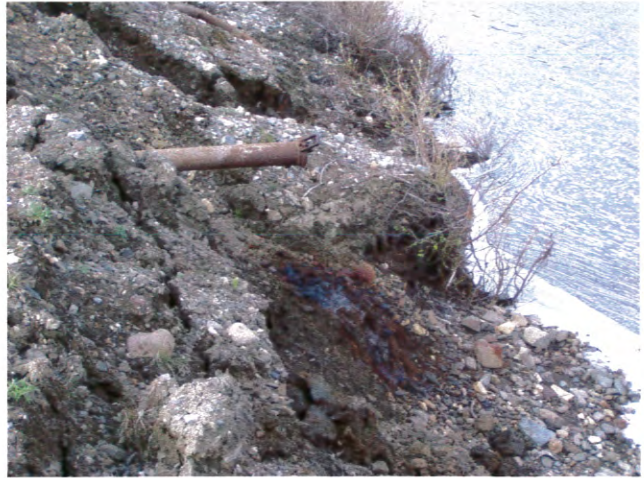
9. Artifact iron pipe as culvert. Note rust-stained soil below outfall.
