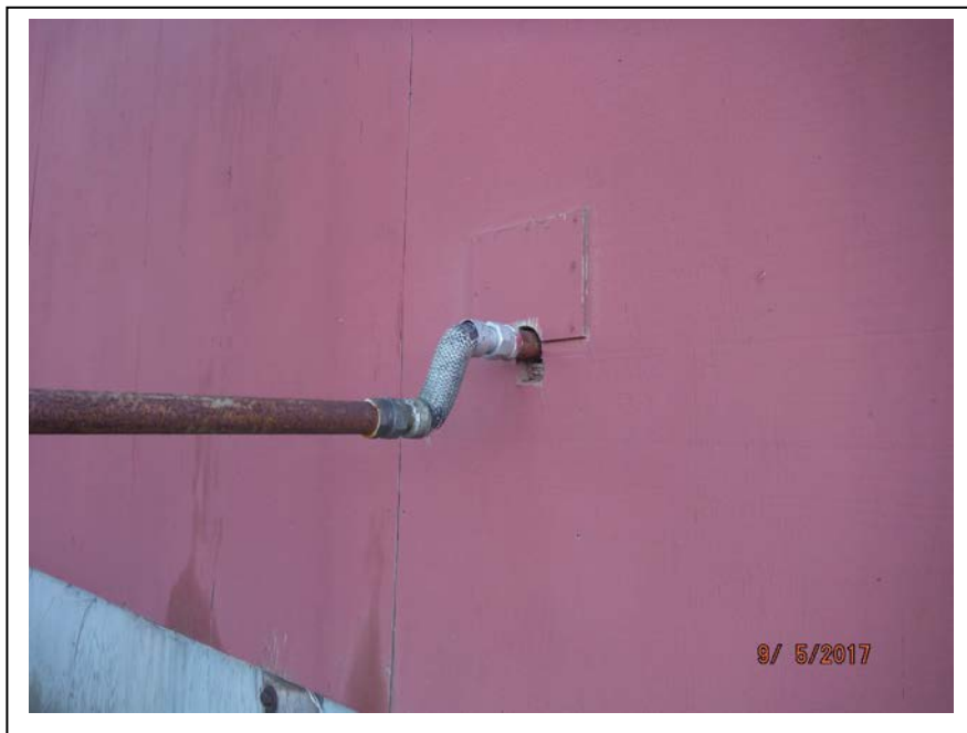
Photograph 2: Product feed piping. (September 5, 2017)
