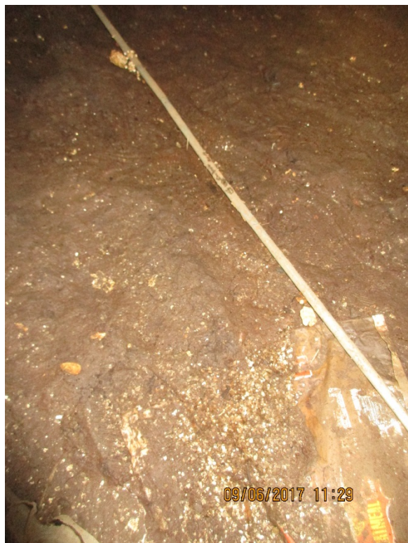
Photo 16: Loose-fill asbestos-containing Vermiculite insulation in soils under building.
