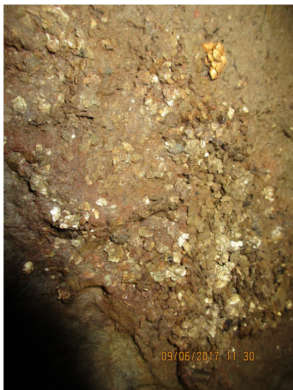
Photo 17: Close-up of asbestos-containing loose-fill Vermiculite insulation in soils under building.
