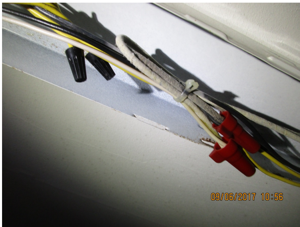
Photo 8: Asbestos-containing high temperature wiring insulation in light fixture.
