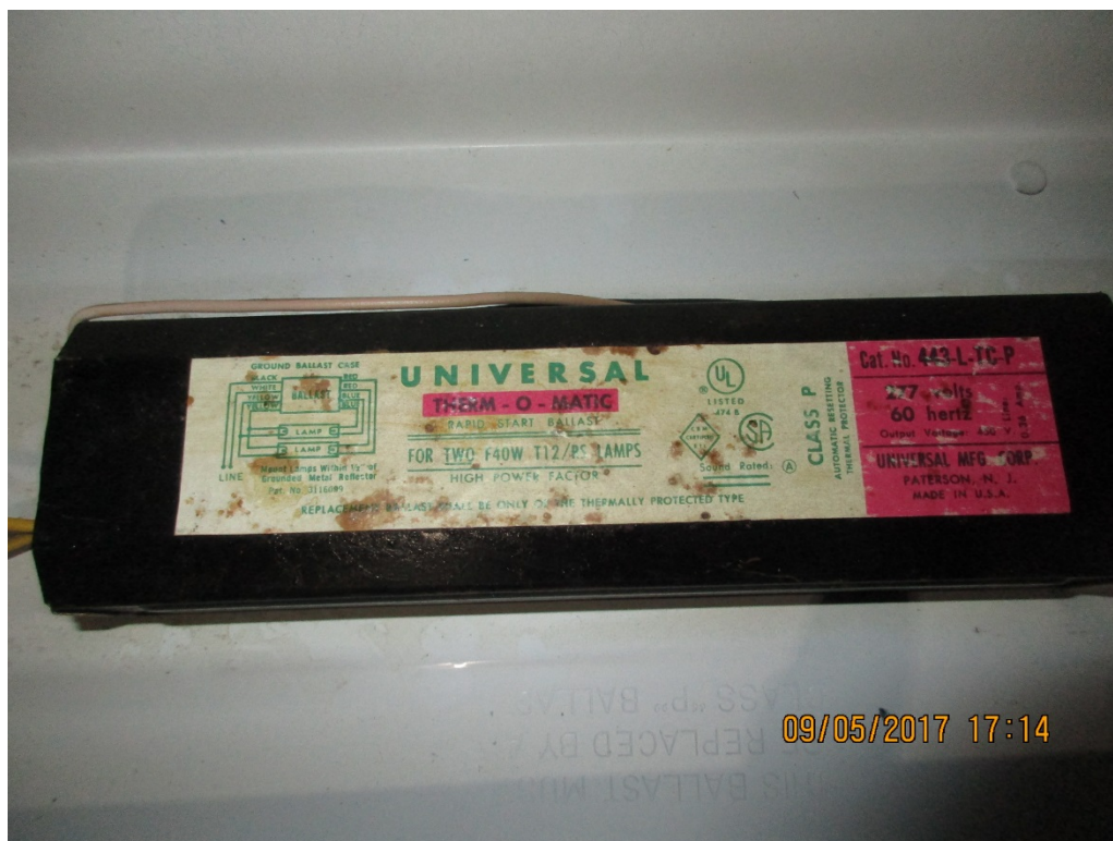
Photo 19: PCB-containing light ballast.
