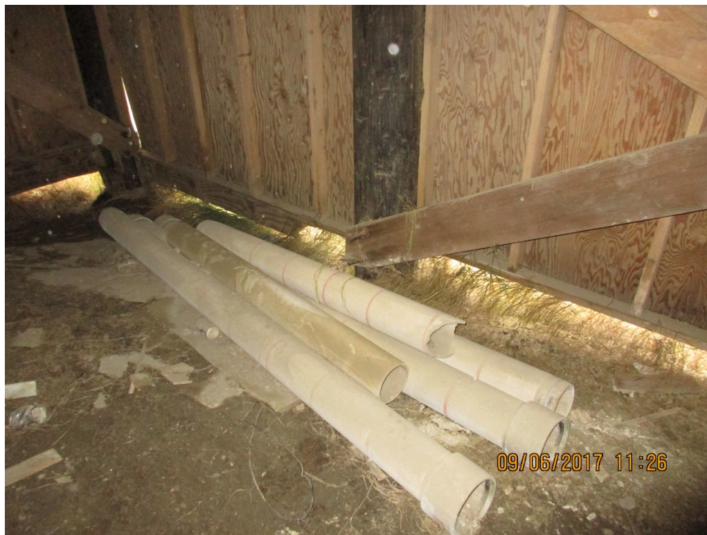
Photo 14: Loose pile of asbestos-containing "Transite" piping under building.
