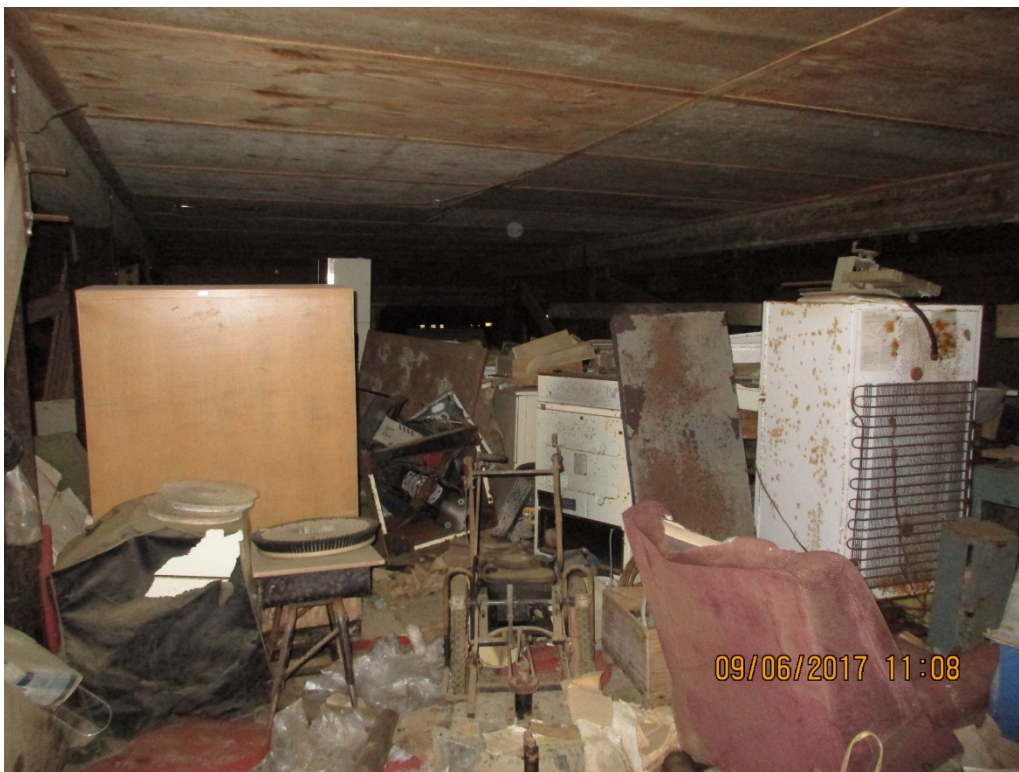
Photo 2: View under Gym showing typical condition of the underside of the building.
