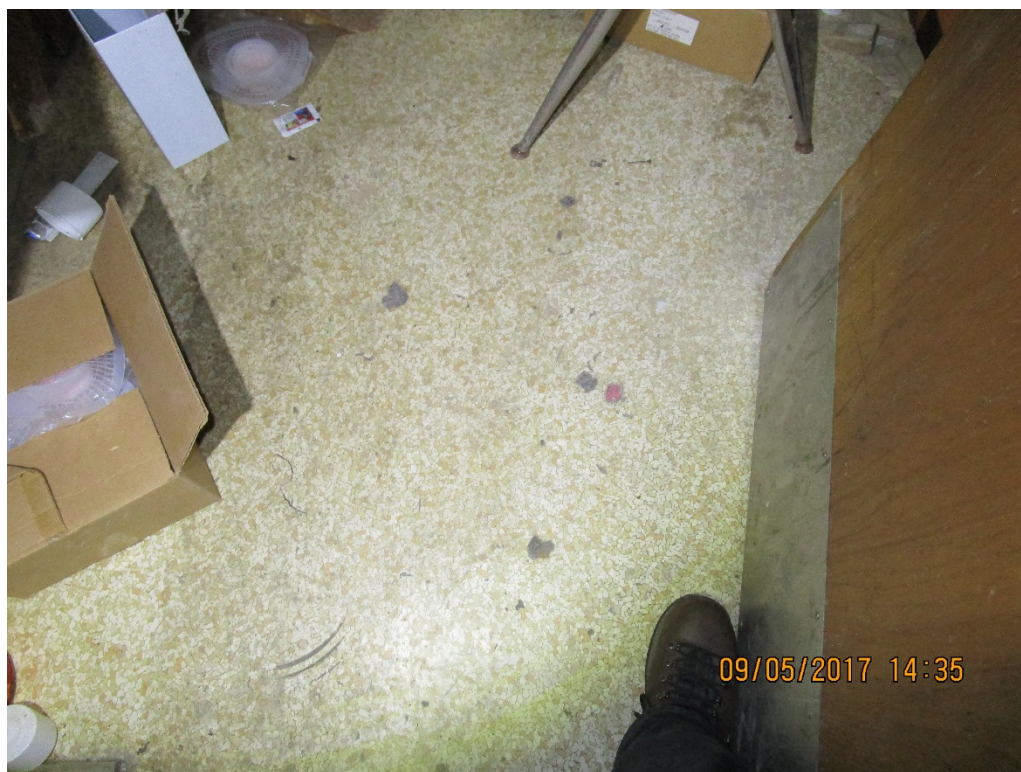
Photo 5: One pattern of asbestos-containing sheet vinyl.
