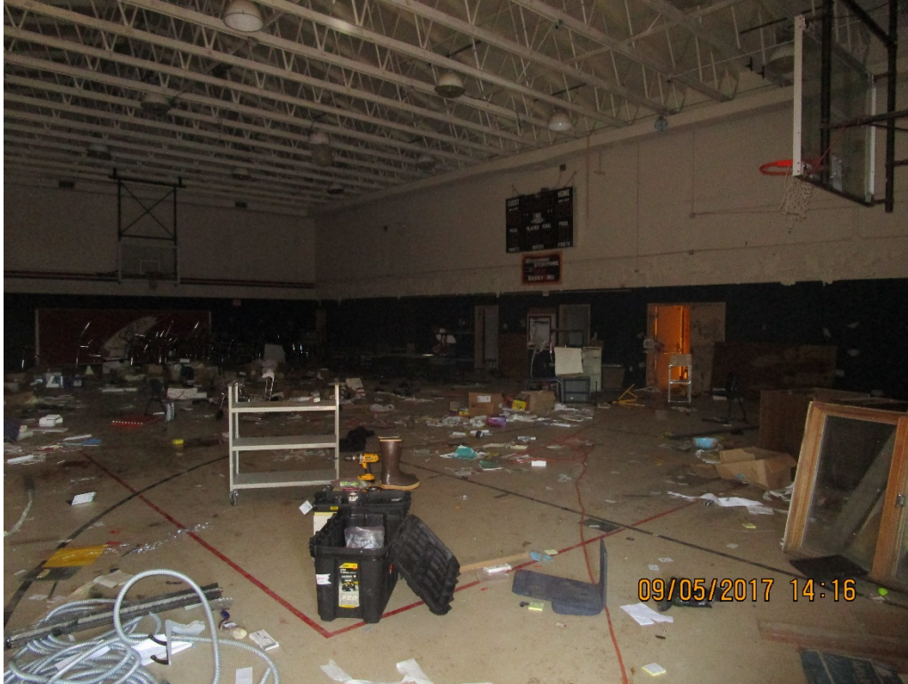
Photo 1: View of Gym showing typical conditions and stored materials in the interior of the building.
