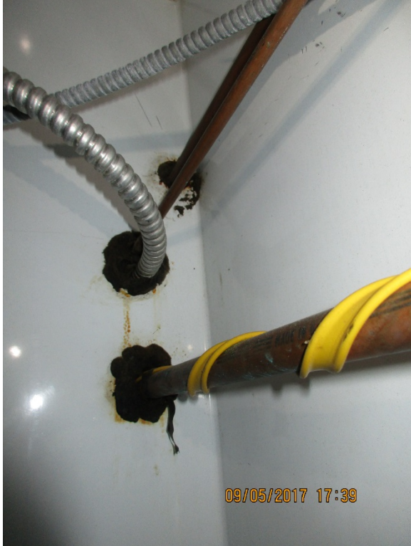
Photo 9: Asbestos-containing penetration putties on refrigerant lines in walk-in freezer in Kitchen.
