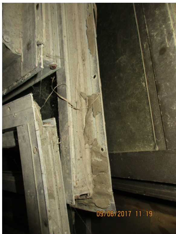
Photo 13: Close-up view of asbestos-containing window putties and sealants
