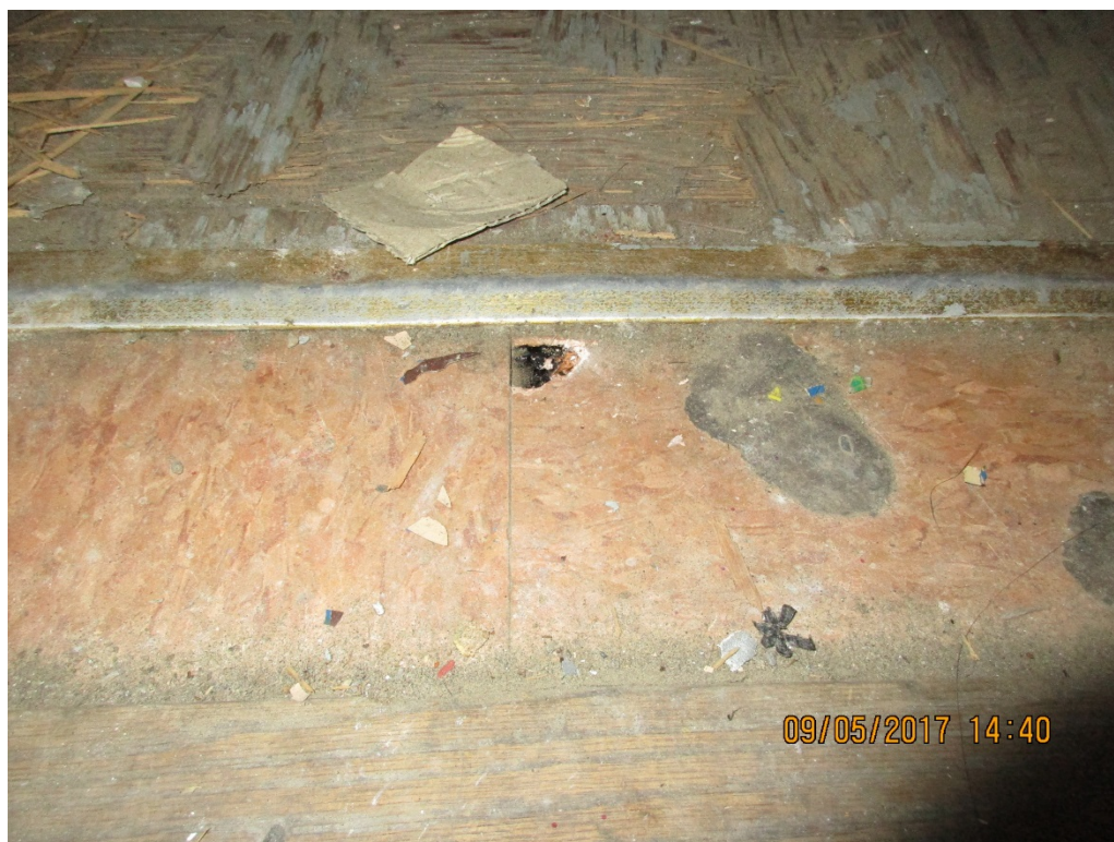
Photo 7: Asbestos-containing black floor tile mastic under vinyl floor tiles under rubber floor in Gym.
