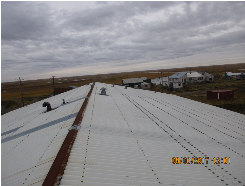
Photo 10: Asbestos-containing patch tars on ridge vent, equipment, and screw heads.
