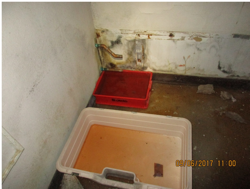
Photo 20: Loose containers of heating system glycol inside the building.
