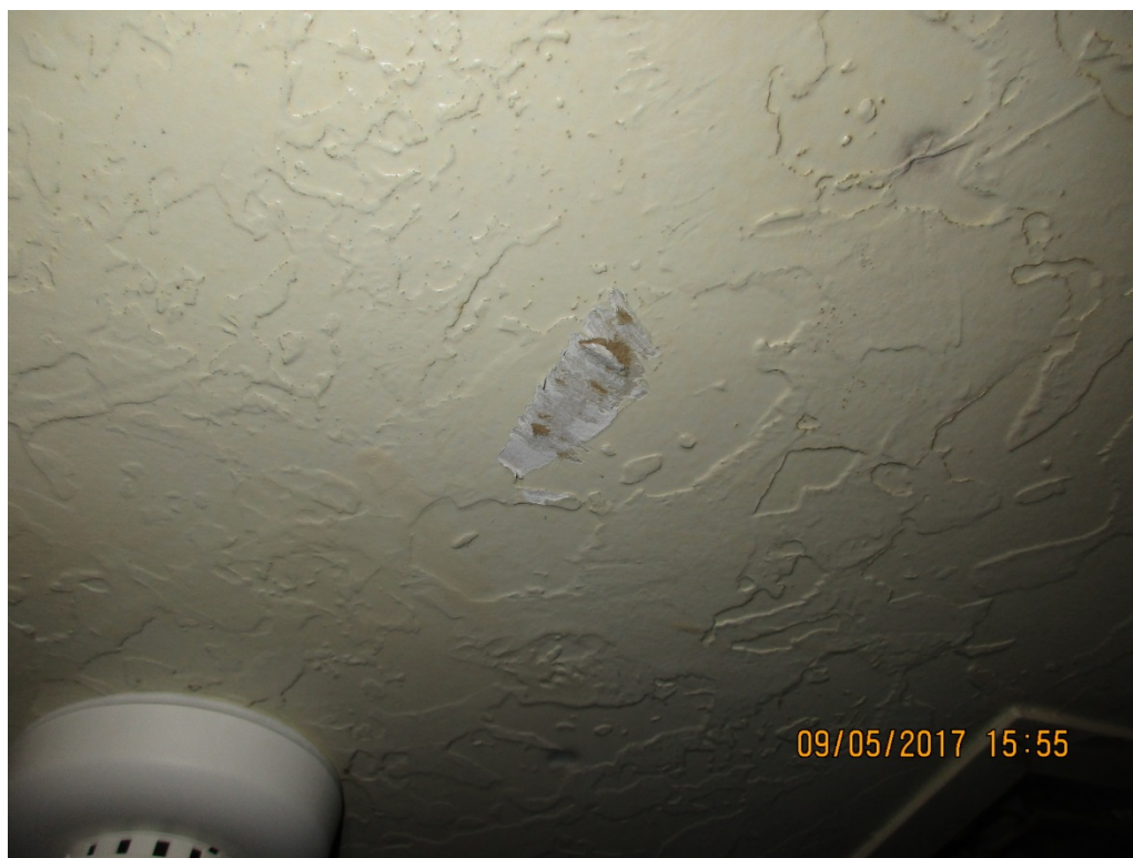
Photo 4: Asbestos-containing troweled-on ceiling texture.
