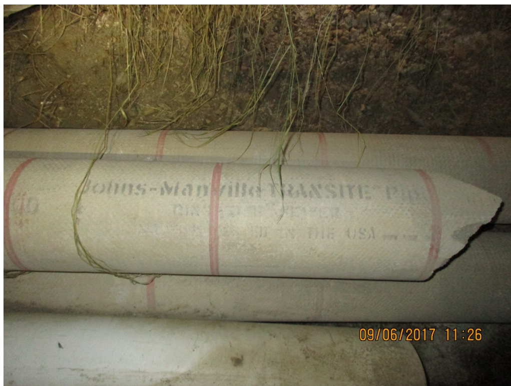
Photo 15: Close-up of loose pile of asbestos-containing "Transite" piping under building.
