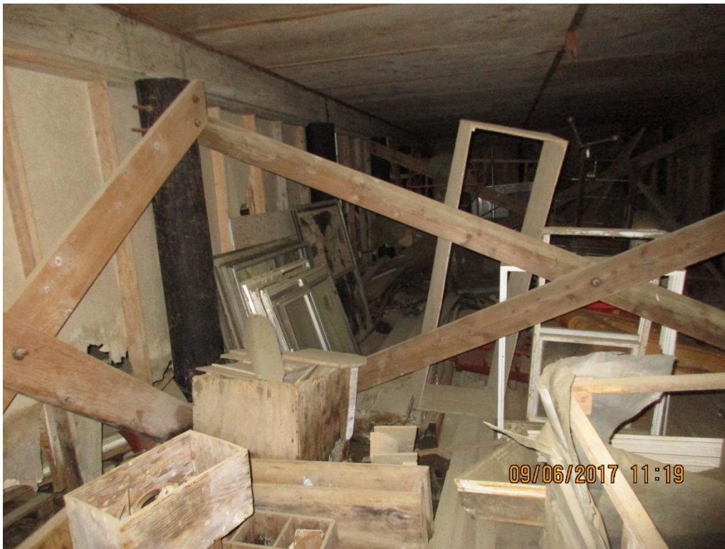
Photo 12: Loose pile of old windows with asbestos-containing window putties under building.
