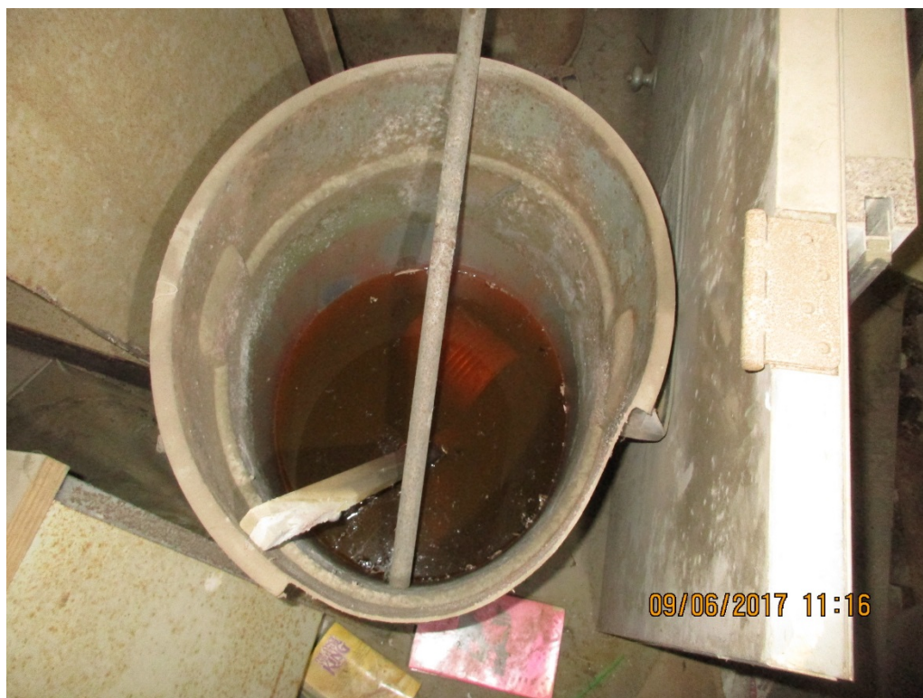
Photo 21: Loose container of heating system glycol under building.
