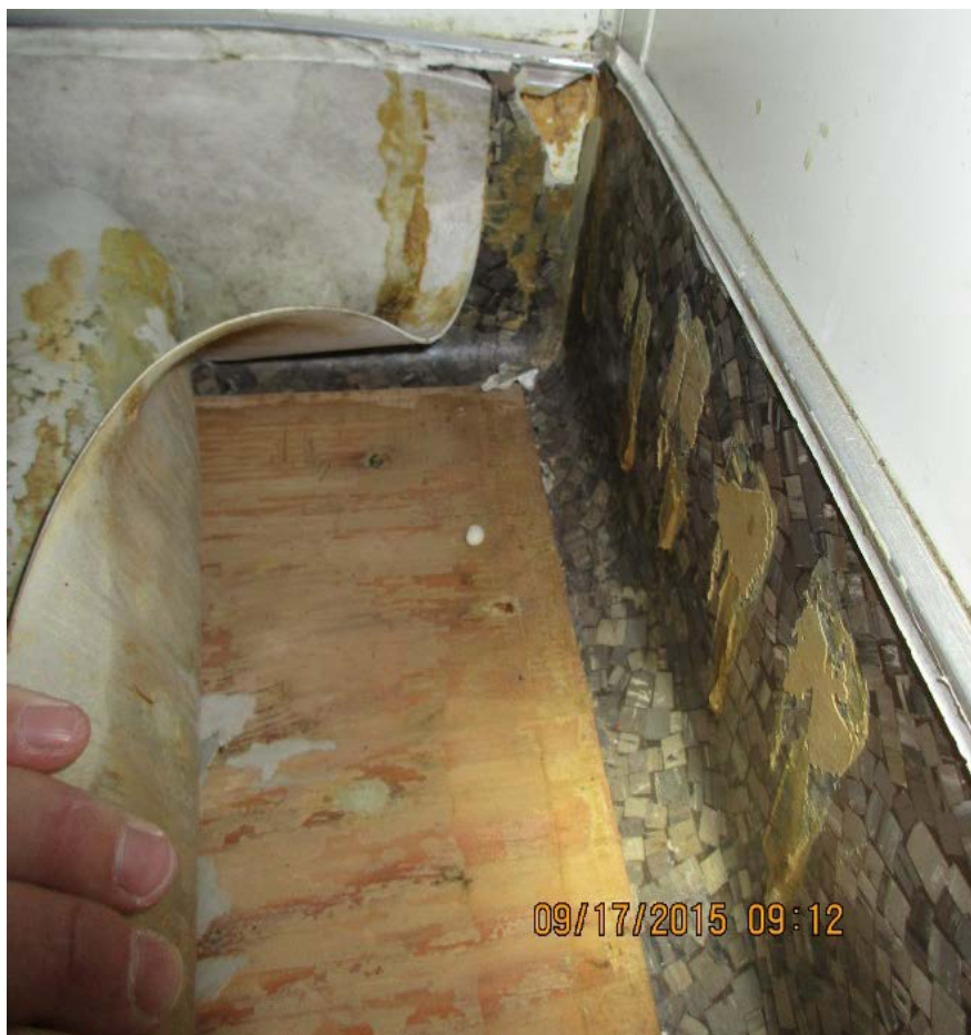
Example of asbestos-containing sheet vinyl concealed under newer non-asbestos sheet vinyl and plywood in the Boy's Bathroom in the Main School Building.
