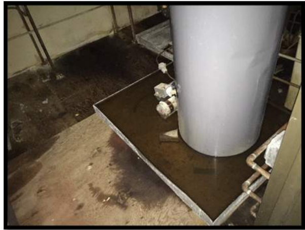
26. Mechanical Room Roof Leak – 1
