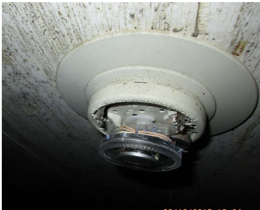
Thermostat with mercury filled ampule in Teacher Housing Unit 1. Note mold on wood wall finish.
