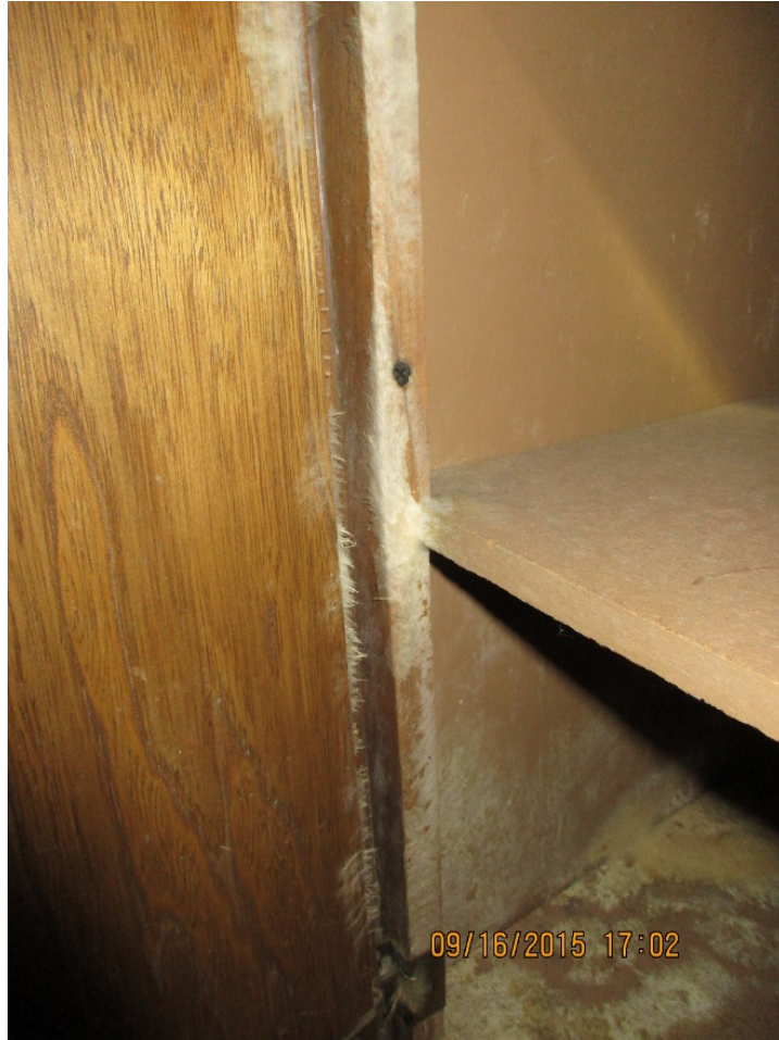
Fungal growth on cabinetry in Kitchen in Teacher Housing Unit 2.
