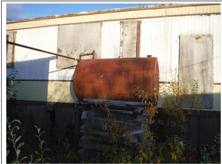
Photo 13: Looking east at AST10 located on the west side of a Teacher Housing Building. (September 16, 2015)
