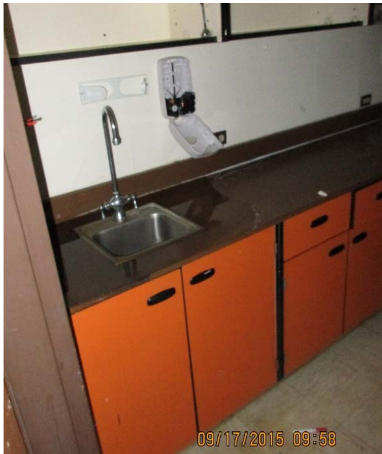
Standing water on countertop in Kitchen in the Main School Building. The source of the water appears to be from the roof leak in the Mechanical Room above.
