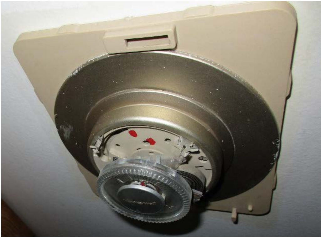
Typical example of a thermostat with a mercury filled ampule in the Main School Building.
