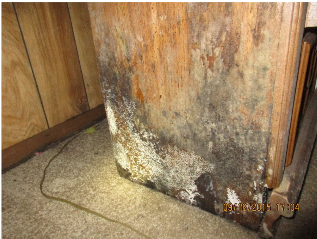
Water damage and fungal growth on loose furniture in Teacher Housing Unit 2.
