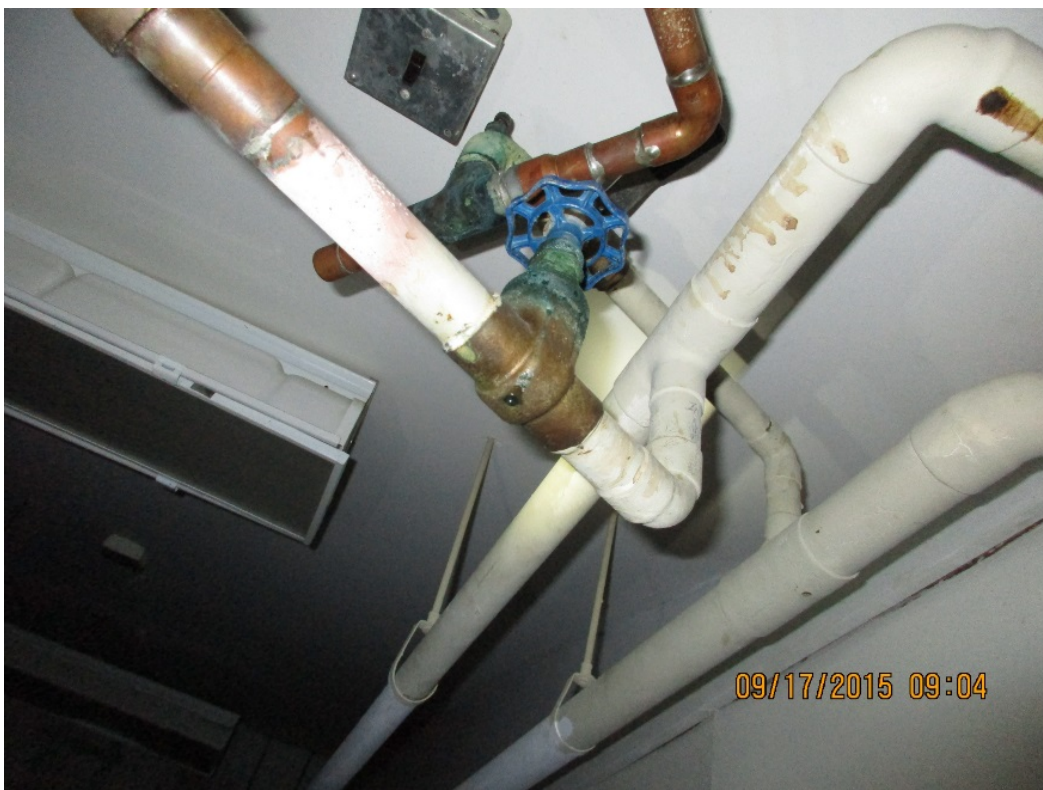
Further evidence of past leaking pipes in classroom on south side of Main School Building.
