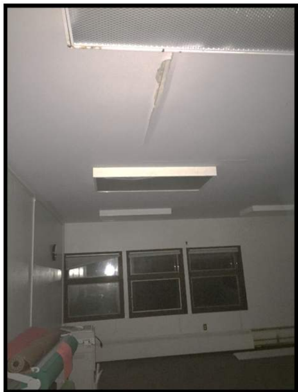
28. Ceiling Water Damage at Corridor 106
