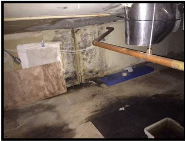
25. Mechanical Room Roof Leak – 3
