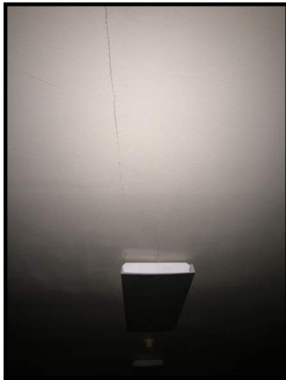
31. Ceiling Sheetrock Damage at North Half of Library
