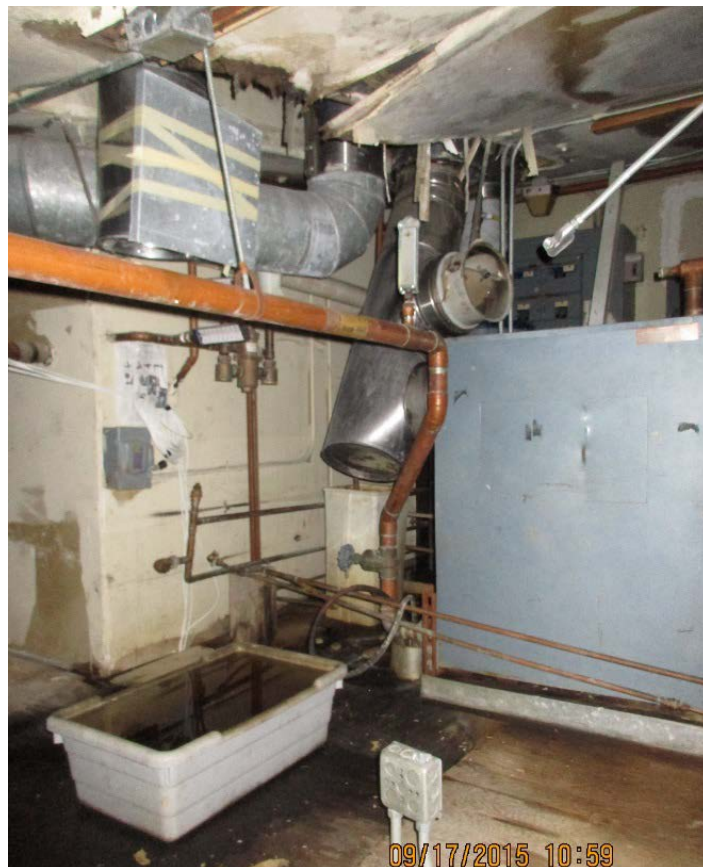
Damaged ceiling in the Main School Building Mechanical Room from active roof leaks above. Note bucket full of water that has overflowed causing more water damage.
