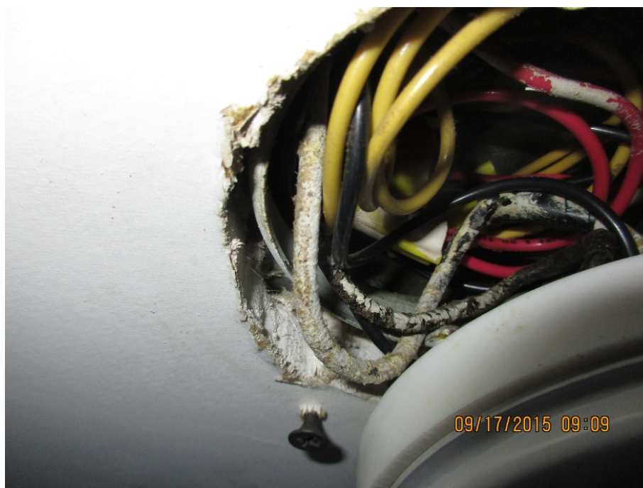
Example of asbestos-containing wire insulation at a heat detector in the Janitor's Closet in the Main School Building.
