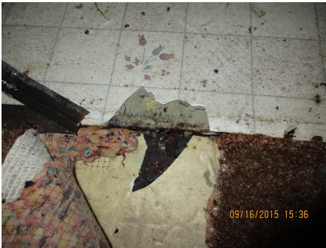
Looking under sheet vinyl in Teacher Housing Unit 1. Note plywood subfloor saturated with water.
