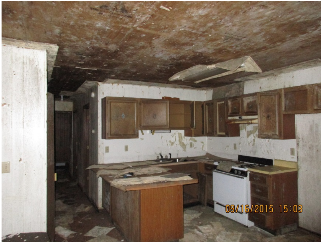
View of Kitchen in Teacher Housing Unit 1. Note extensive water damage and mold on virtually all surfaces.
