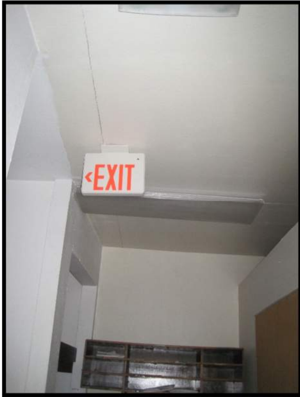
29. Ceiling Sheetrock Damage at Library Entry
