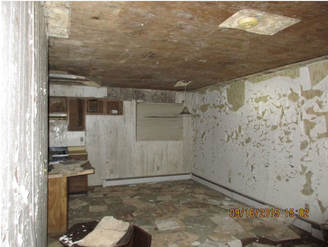
View of Living Room area in Teacher Housing Unit 1. Note extensive water damage and mold on virtually all surfaces.
