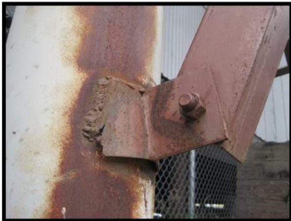
15. Cracked Weld at Stair Connection
