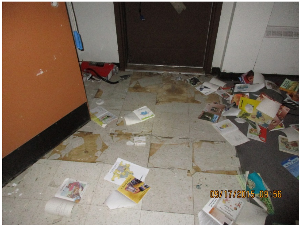
Example of damaged asbestos-containing floor tiles in the large classroom at the southeast corner of the Main School Building. Damage is caused by a combination of water damage, foot traffic, and abrasion from the doors being opened and closed.
