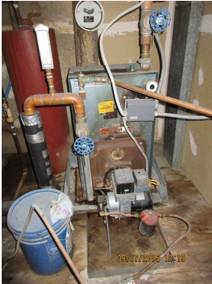
Small Mechanical Room in the 1984 addition. Note water stained floor and wall, and mineral build up on boiler flue. There did not appear to be an active leak at the time of inspection.
