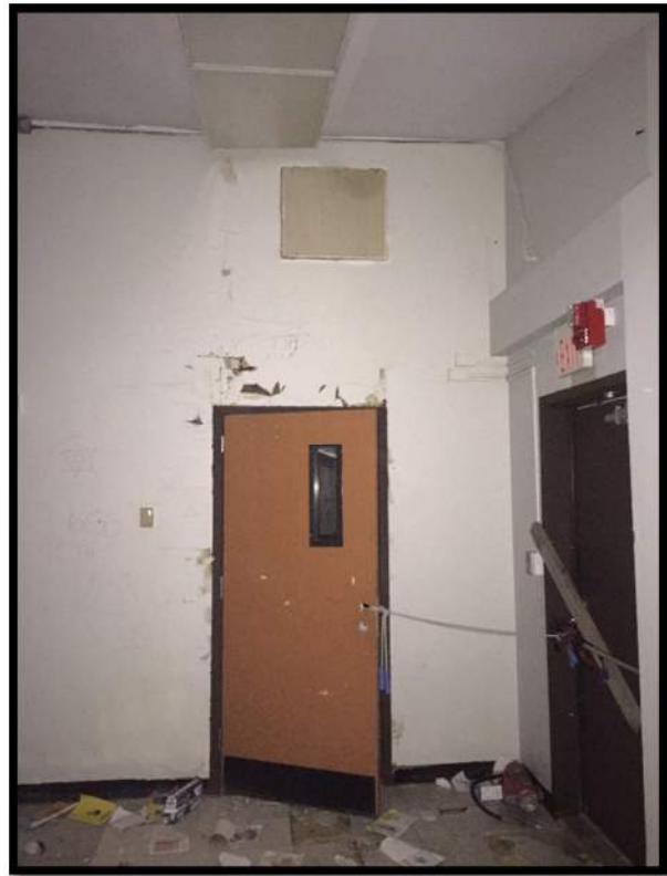
22. Water Damage at NE Corner of Academic Room
