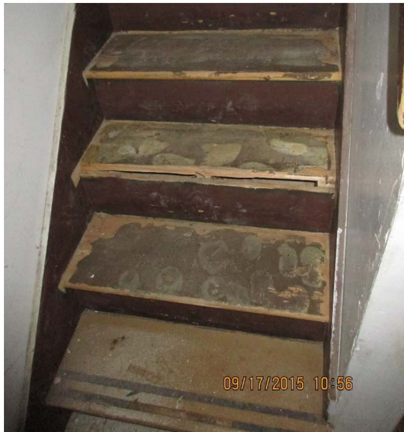
Example of damaged asbestos-containing stair treads at stairway that leads from the Kitchen to the Mechanical Room in the Main School Building.
