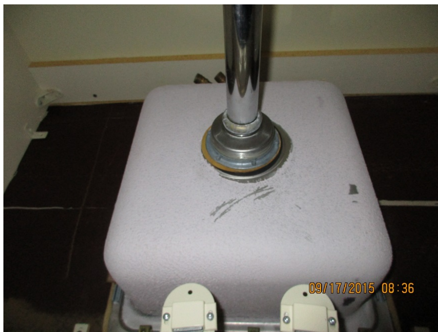
Typical stainless steel sink with asbestos-containing undercoating in the Main School Building.
