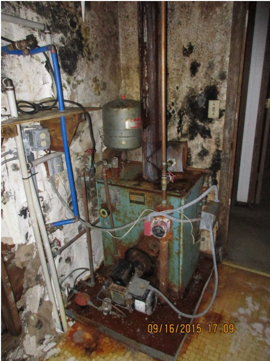
Boiler in Teacher Housing Unit 2. Note boiler drip pan is full of water, water damage to floors, walls, and ceiling, and the extensive mold growth.
