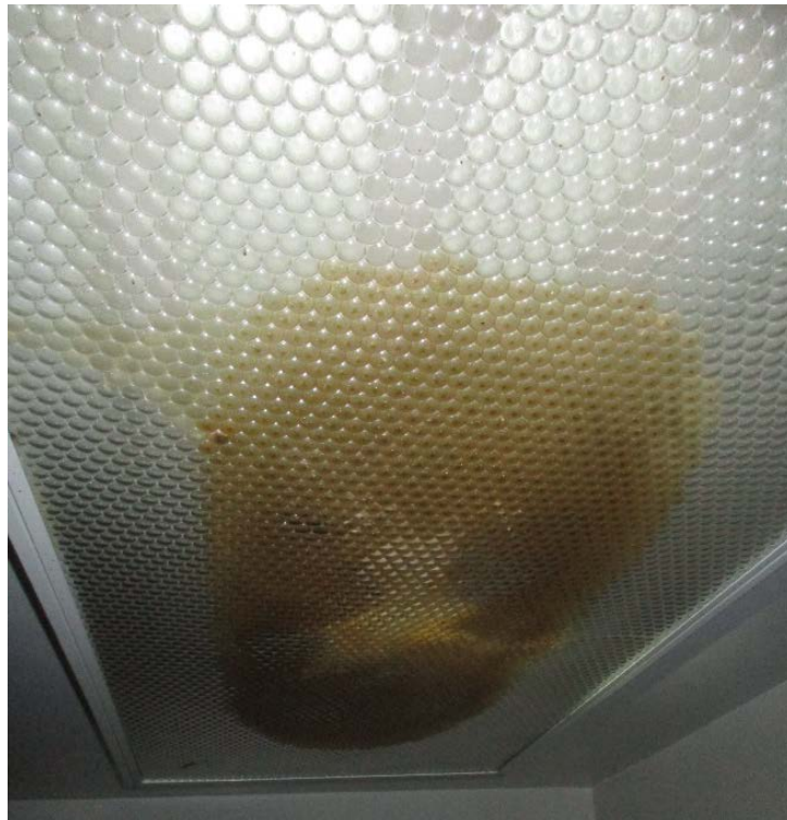
Water damaged light fixture in Kitchen area in large classroom at the southeast corner of the Main School Building. The source of water appears to be from the leaking roof and overflowing catch buckets in the Mechanical Room above.
