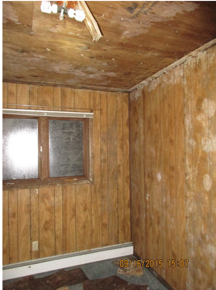
Water damaged floors, walls, and ceiling with mold in a bedroom in Teacher Housing Unit 1. Note moisture on the inside face of the window glass.
