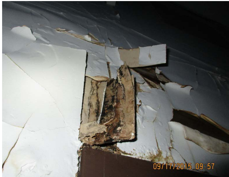
Close up of damaged wall above door leading to Kitchen in large classroom at southeast corner of Main School Building. Note the black mold and deteriorated gypsum board. The source of the water appears to be from the roof leak in the Mechanical Room above.
