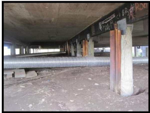
12. Rolled GLB & Missing Pile Saddle Bolts
