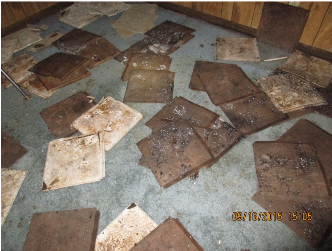
Typical bedroom in Teacher Housing Unit 1 with water damaged and moldy ceiling tiles and other surfaces.
