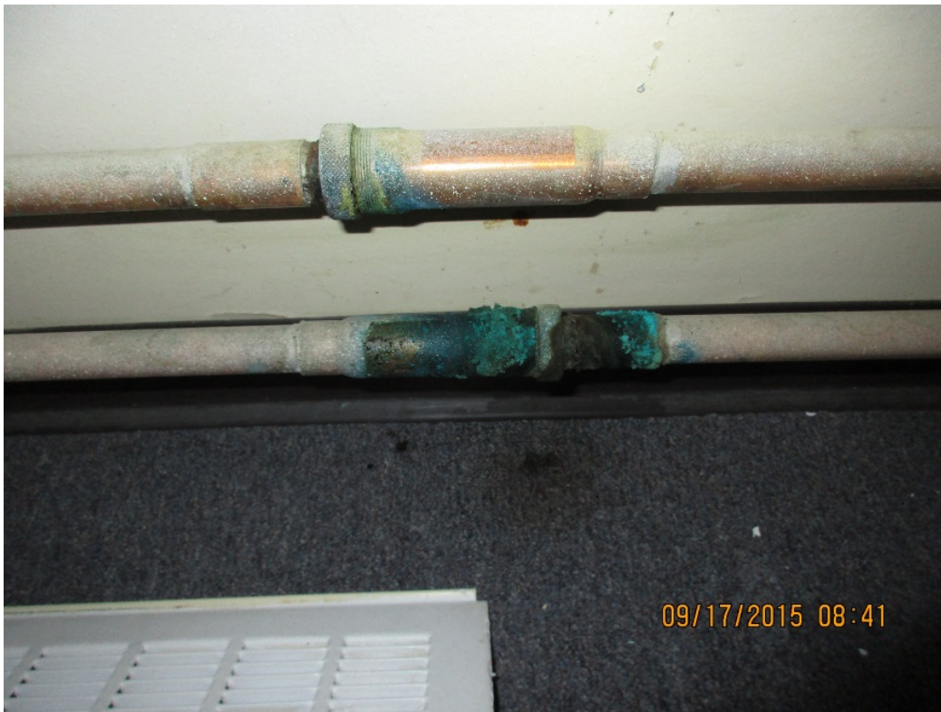
Evidence of past leaking heat piping in classroom on north side of Main School Building. Note water droplets on pipe.
