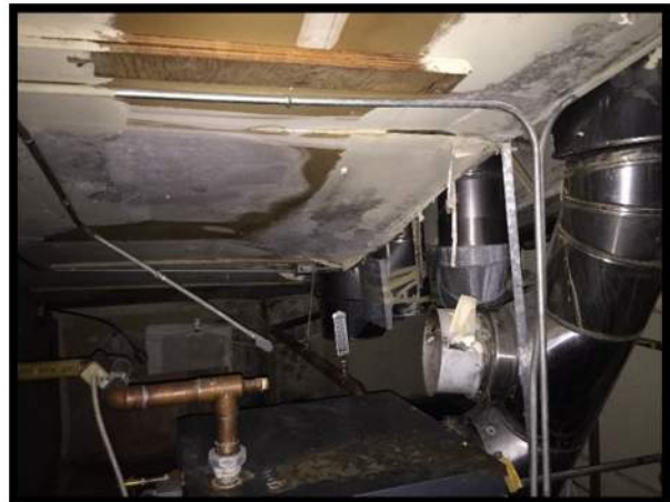
24. Mechanical Room Roof Leak – 2
