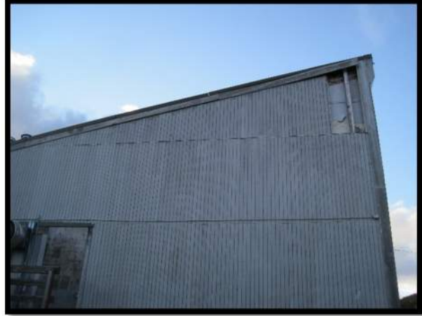
2. Missing Exterior Siding – NE Corner Gymnasium
