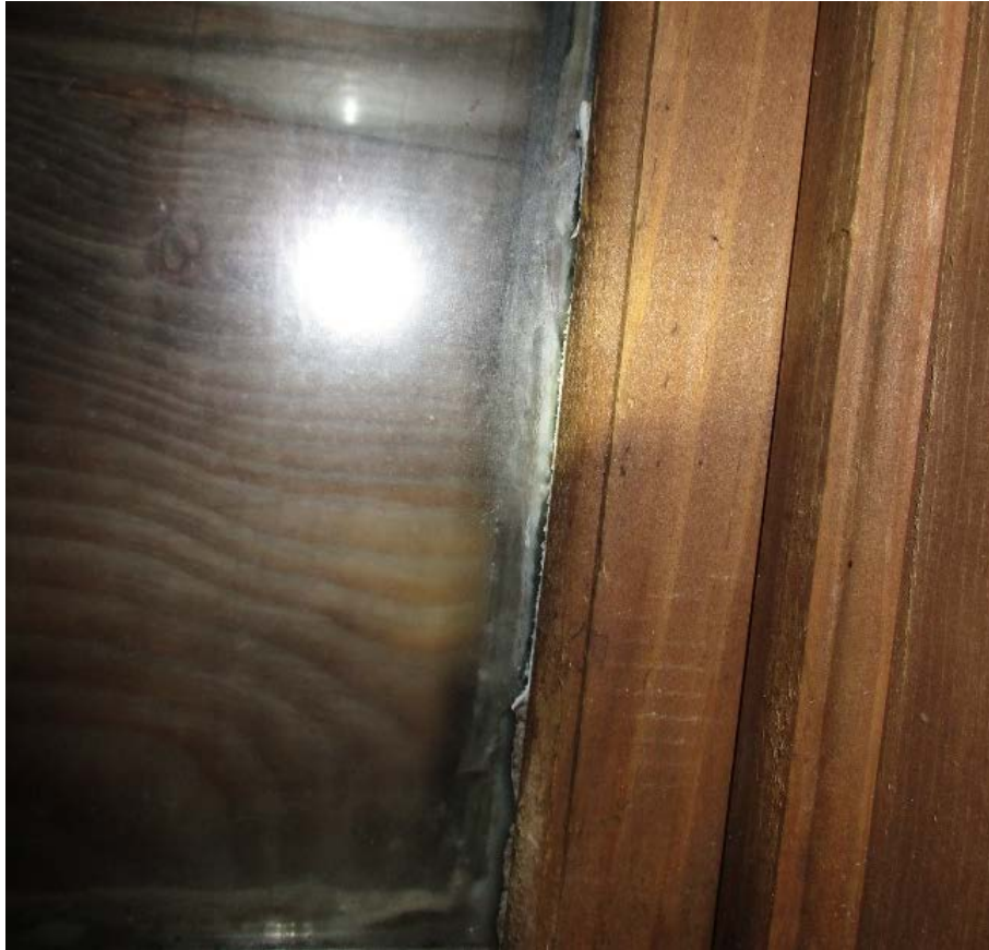
Asbestos-containing window glazing compound on older window in Teacher Housing Unit 1. Teacher Housing Unit 2 similar.
