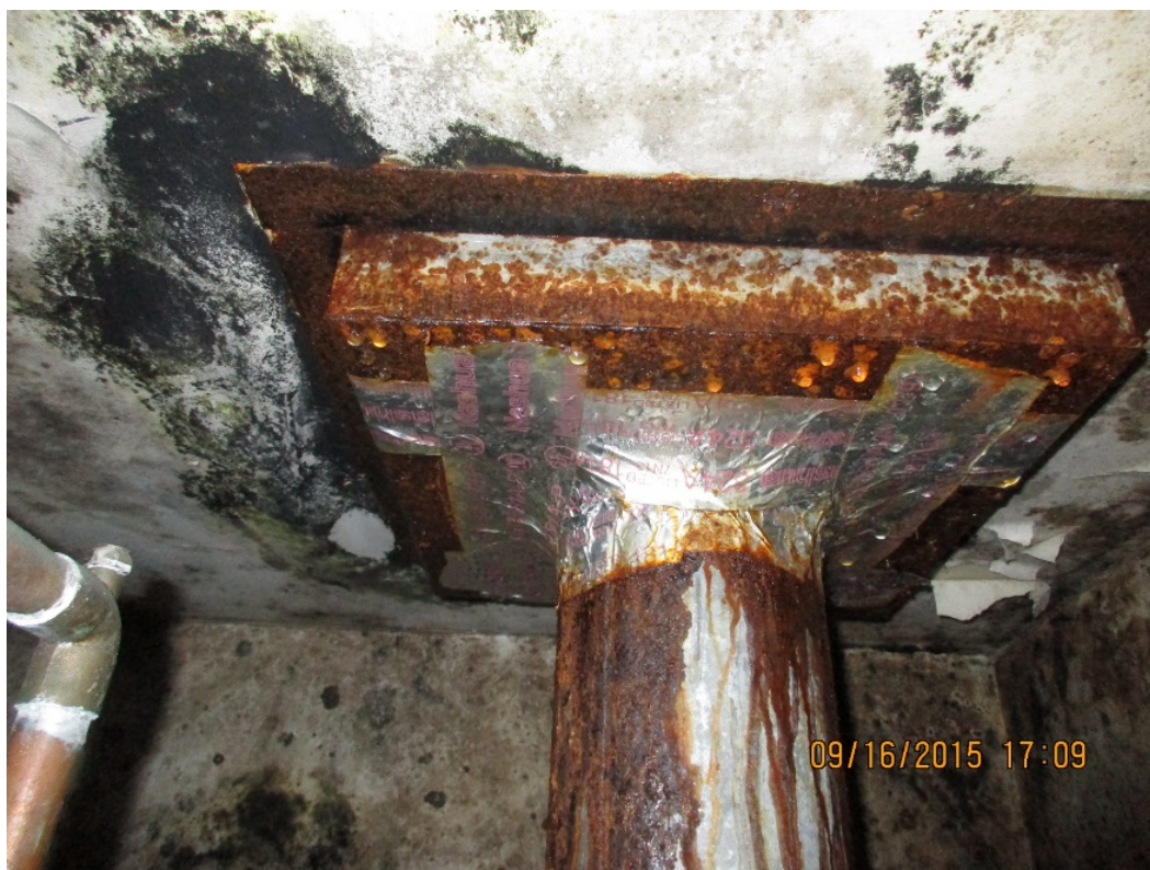
Condensation on boiler flue in Teacher Housing Unit 2. Note water damaged walls and ceiling and mold.
