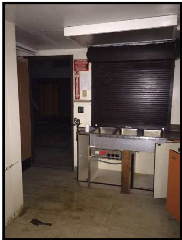
20. Active Leak at Ceiling of Kitchen
