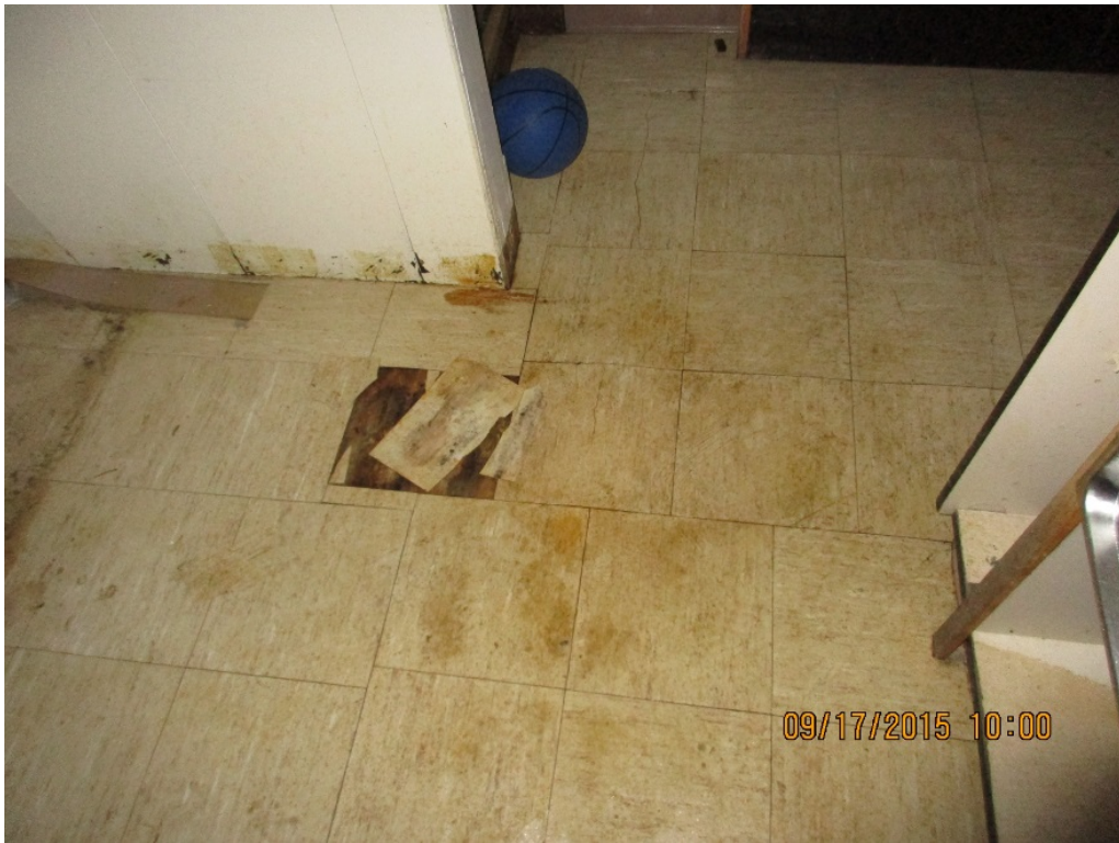
Non-asbestos floor tile damaged by water leaks from above in Kitchen. The source of the water appears to be from the roof leak in the Mechanical Room above.
