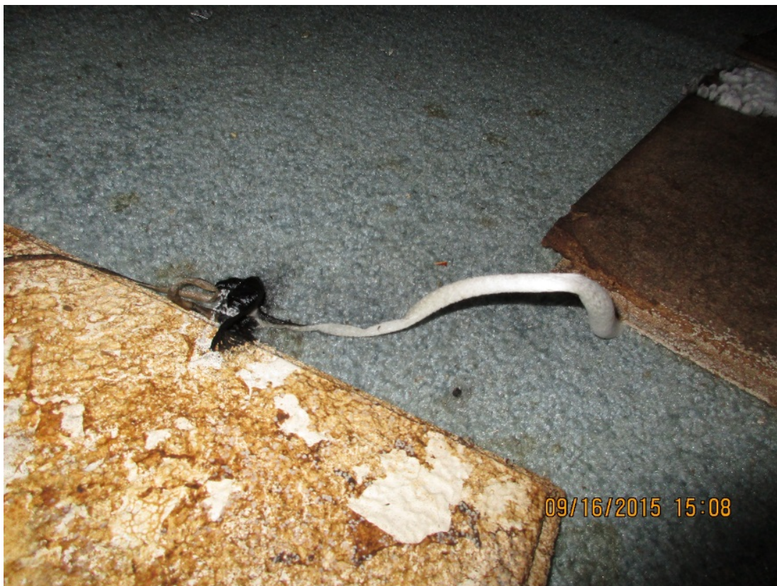
Mushroom growing out of floor with mold on ceiling tile in a bedroom in Teacher Housing Unit 1.
