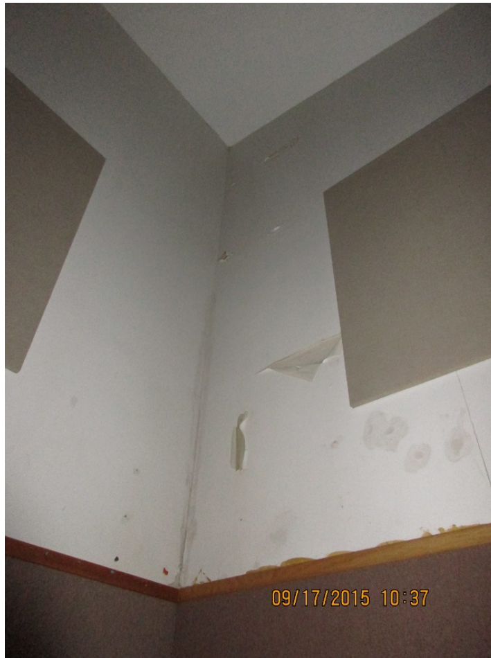
Water damaged wall at northeast corner of Gym. Daylight is visible through cracks at the wall/ceiling connection.
