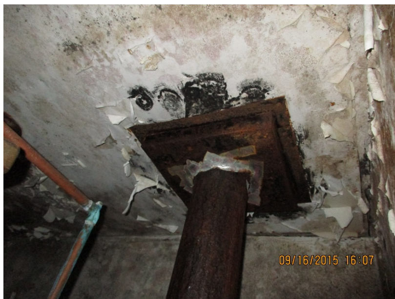
Water damaged ceiling and walls with mold at boiler flue in Teacher Housing Unit 1.
