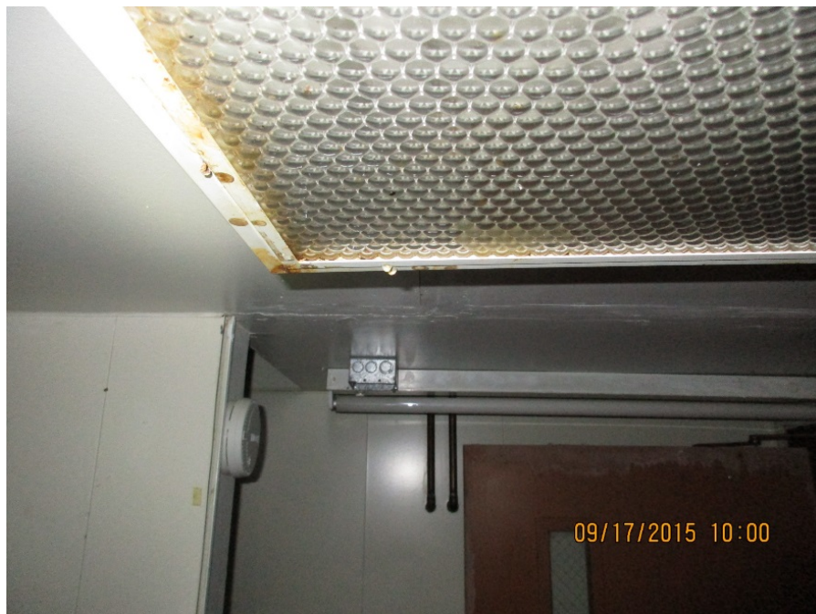
Water leaking out of light fixture in Kitchen in the Main School Building. The source of the water appears to be from the roof leak in the Mechanical Room above.
