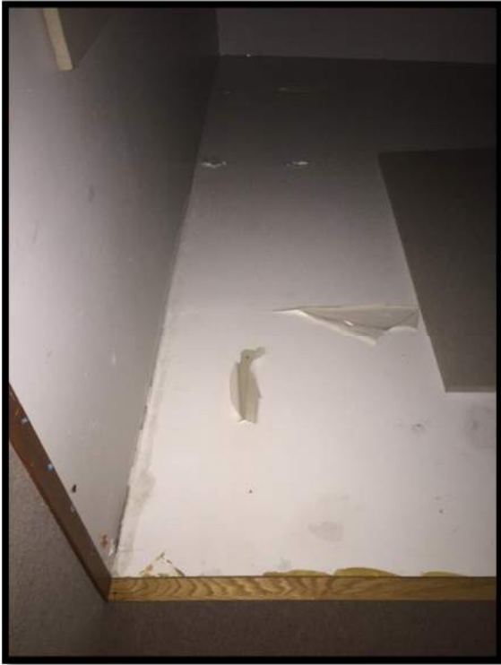
17. Water Damage at Wall of NE Corner of Gymnasium
