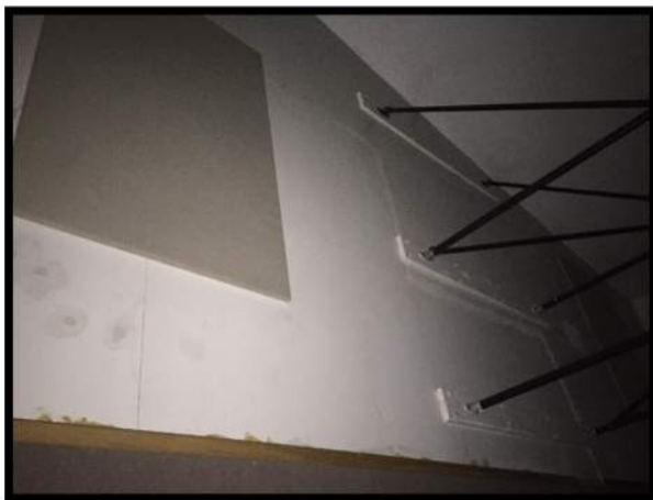
19. Cracks at East Wall of Gymnasium
