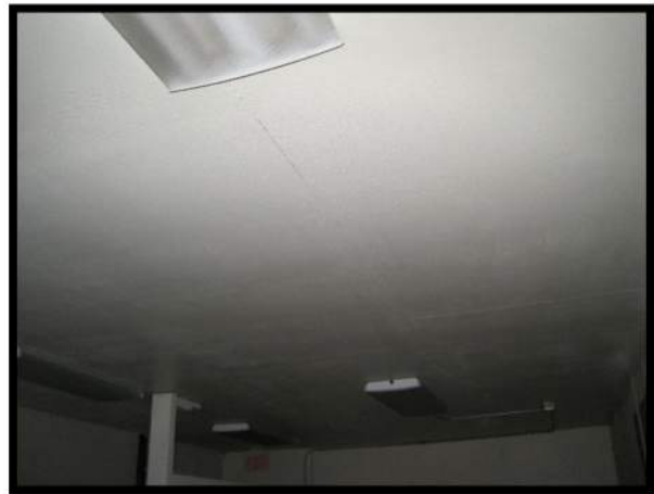
30. Ceiling Sheetrock Damage at North Half of Library – 1
