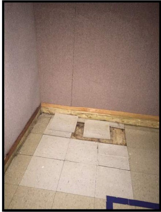
18. Water Damage at Floor of NE Corner of Gymnasium
