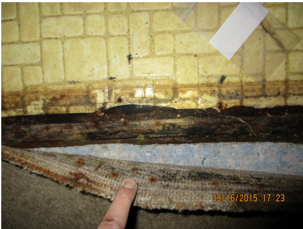
Fungal growth on plywood subfloor in Teacher Housing Unit 2. Note water saturated flooring materials and subfloor.
