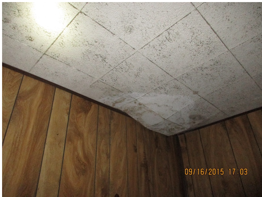
Water damaged ceiling in a bedroom in Teacher Housing Unit 2. Note mold growth on ceiling tiles and walls.
