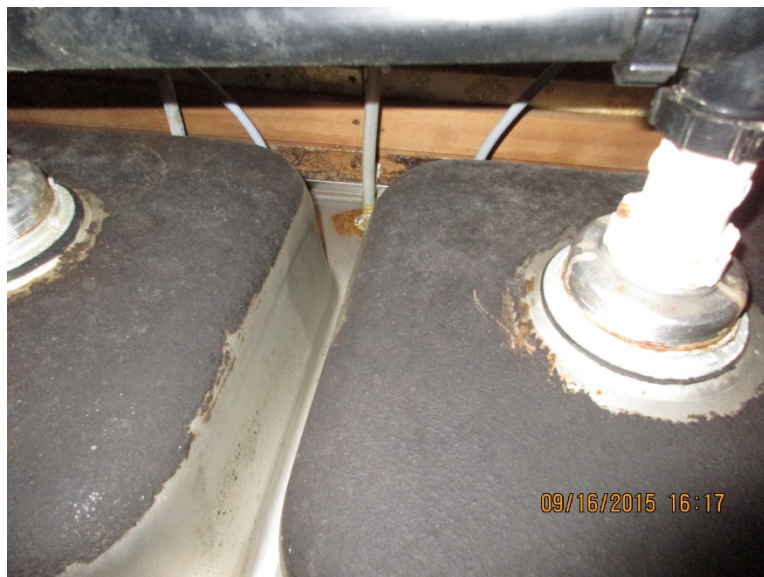
Asbestos-containing sink undercoating on Kitchen sink in Teacher Housing Unit 1. Teacher Housing Unit 2 similar.
