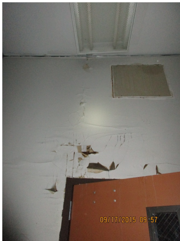
Damaged wall above door leading to Kitchen in large classroom at southeast corner of Main School Building. Note water staining and damaged gypsum board. The source of the water appears to be from the roof leak in the Mechanical Room above.
