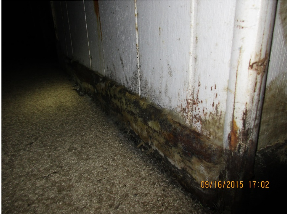
Fungal growth on carpet, base trim, and wood paneling of cabinetry near the Kitchen in Teacher Housing Unit 2.
