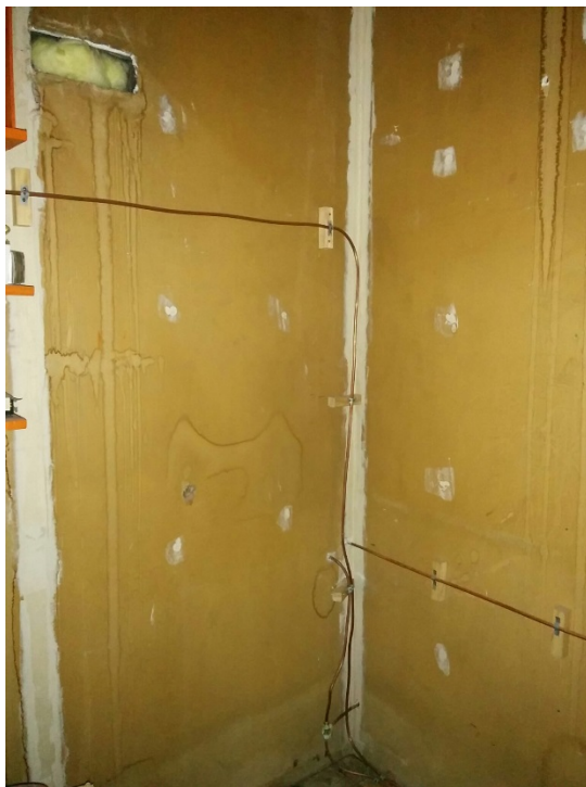
Photo 33 – Joint compound (Room E, sample AS08, 1.2% asbestos)
