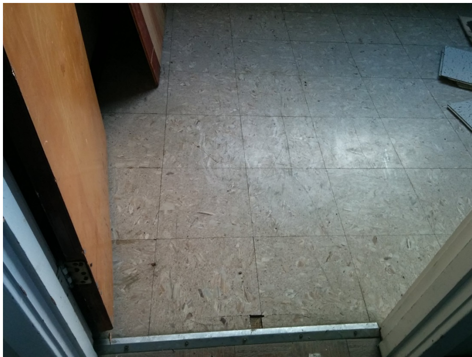
Photo 29 – Tan/brown floor tile (Room A, sample AS02, 1.3% asbestos)
