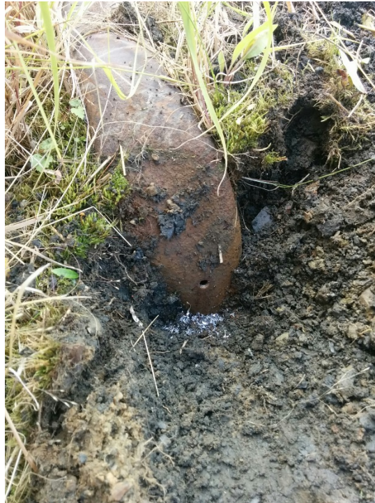
Photo 3 – Bent-over UST fill/vent pipe
