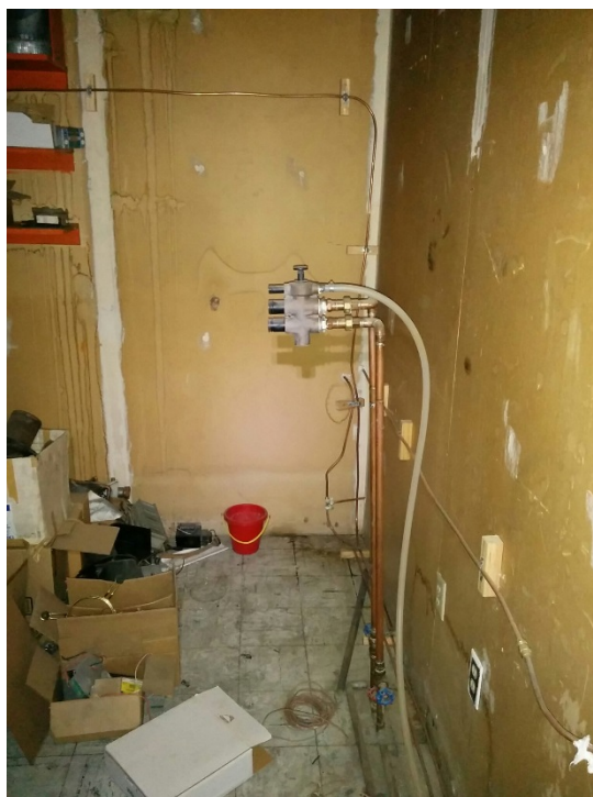
Photo 12 – Corner of furnace room with fuel-affected flooring
