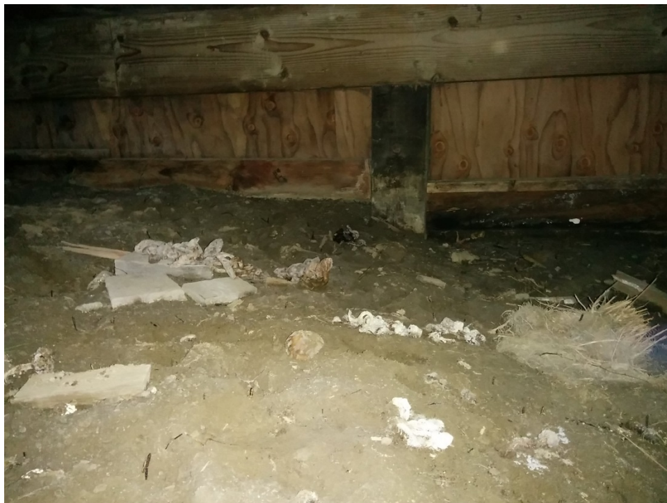
Photo 26 – Building crawlspace – mushrooms growing in soil
