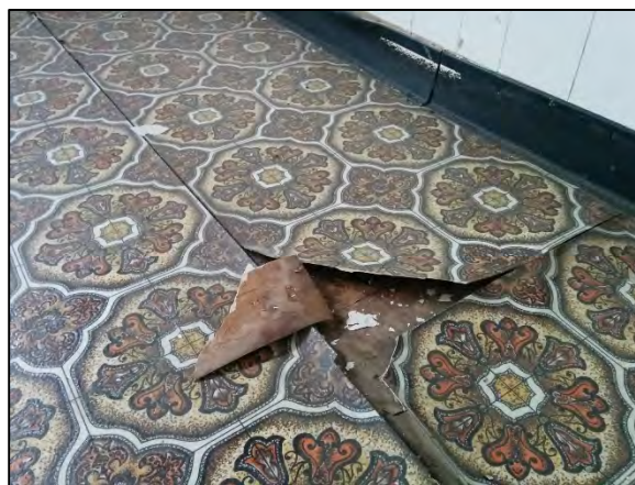
FIGURE 12 – DAMAGED SHEET VINYL (25% ASBESTOS)
