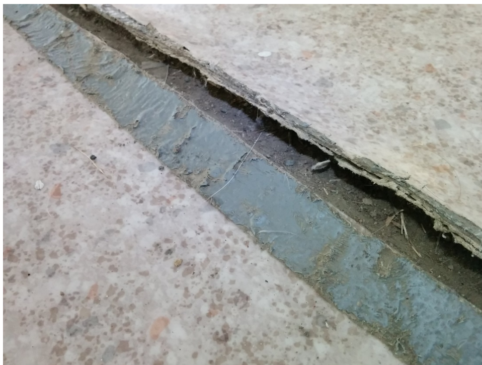
Photo 34 – Tan/black mastic (Room I, Sample AS11, 1.5% asbestos)
