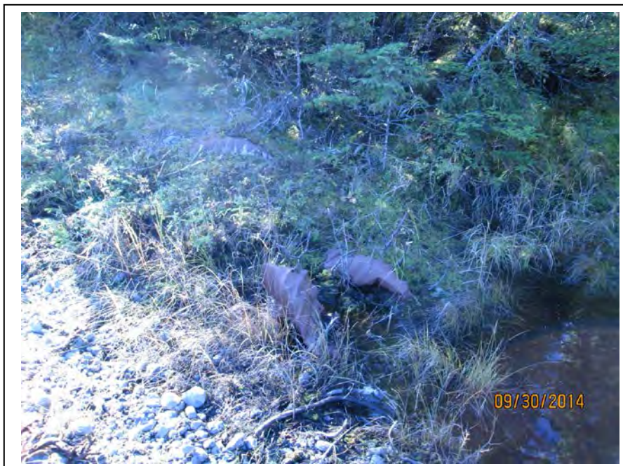
Photo 6: Rusty culverts along Cabin Lake Road (020), looking northwest. (September 30, 2014)
