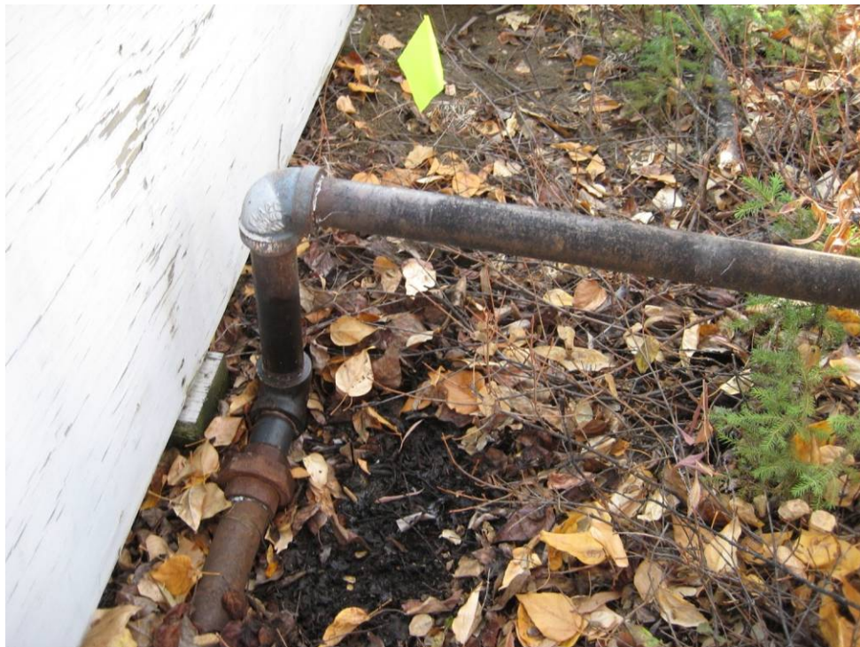
Photograph 4: Leaking coupling near utilidor east of tank farm (September 2009).
