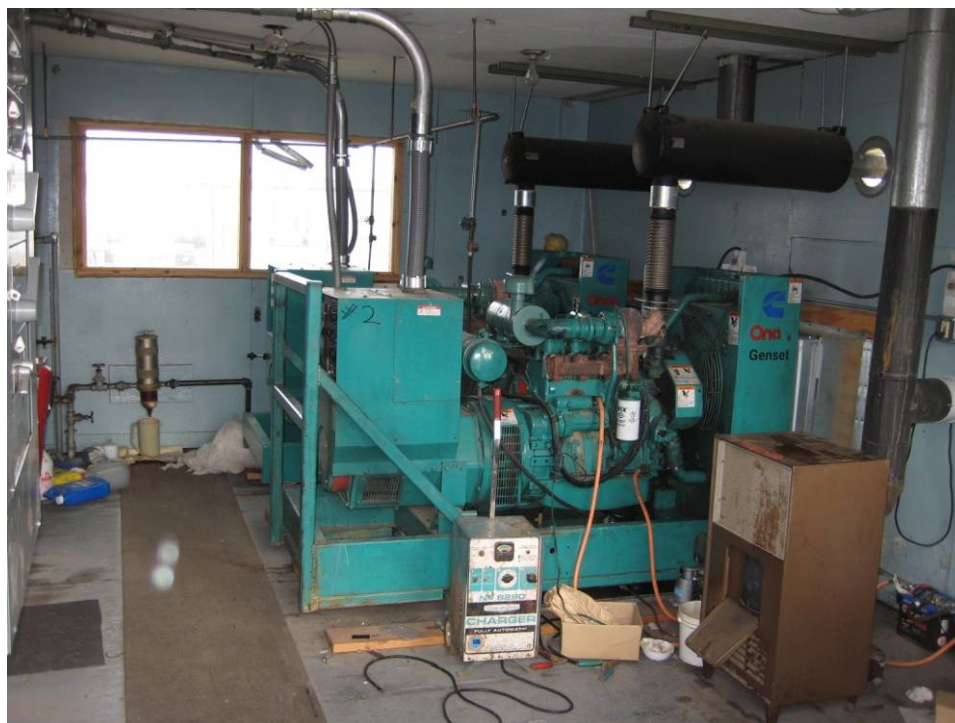
Photograph 8: Inside generator building (September 2009).
