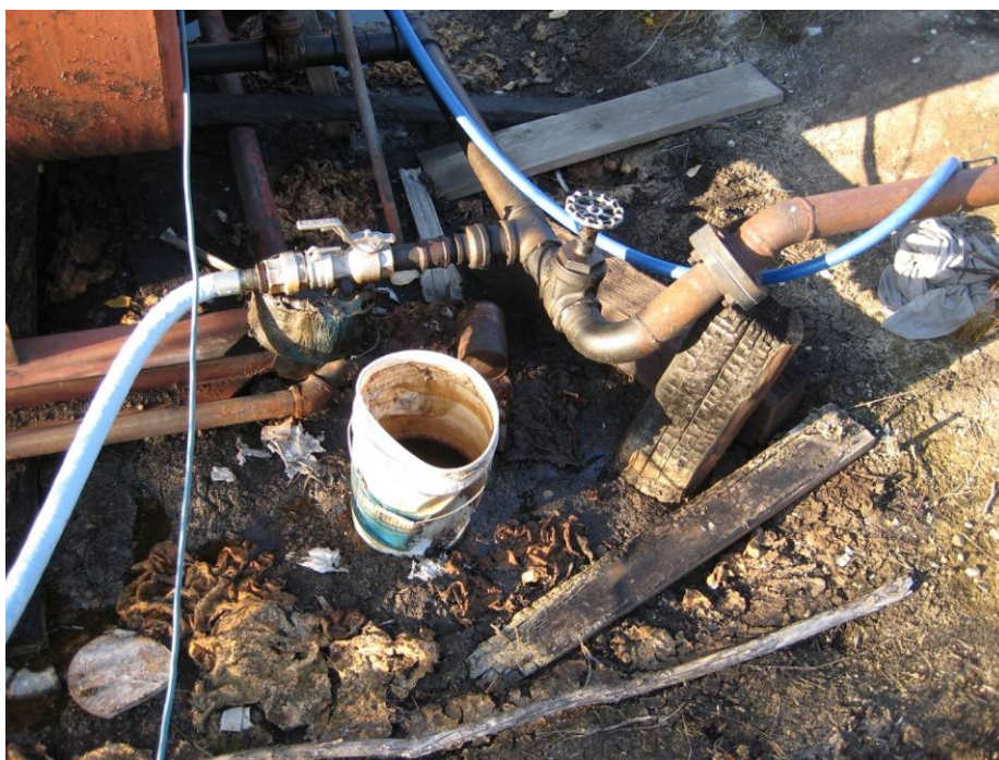
Photograph 3: Leaking pipe fittings at BJU Tank Farm (September 2009).
