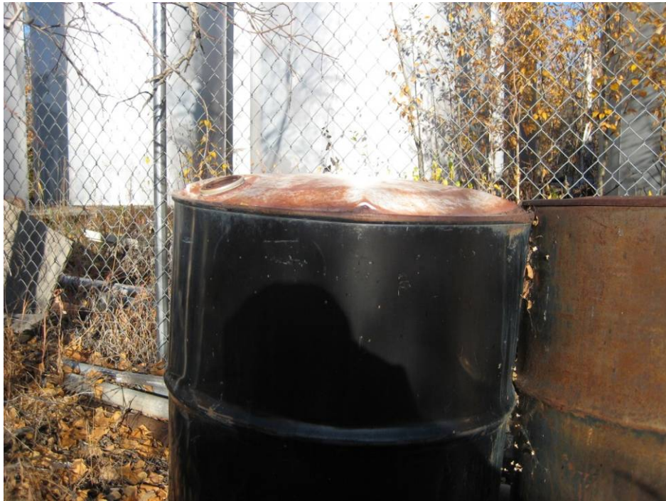
Photograph 3: Drum conditions at the tank farm (September 2009).
