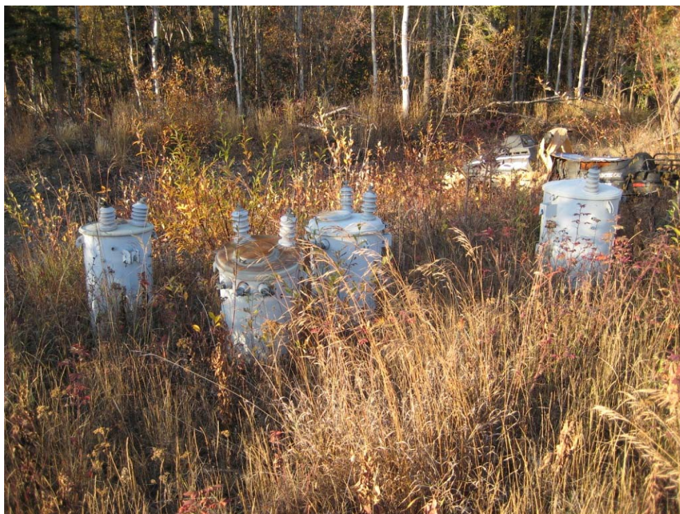
Photograph 7: Transformer storage west of BJU Tank Farm (September 2009).
