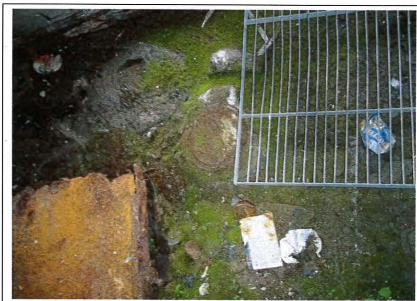
Photo H-20: Representative floor of a ground floor room covered with moss and other litter/debris. (September 8, 2014)
