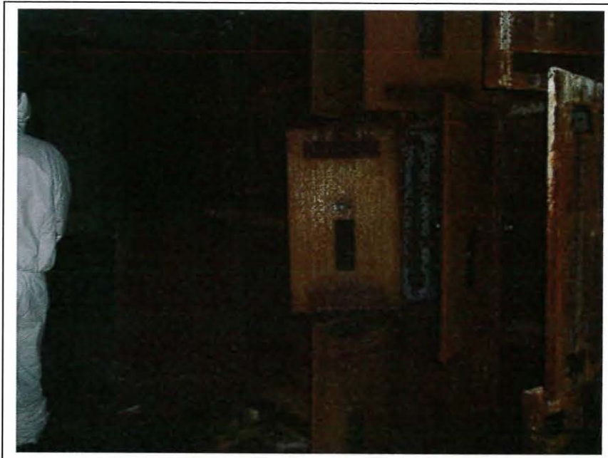
Photo H-9: Distribution panels in the Section A electrical distribution room. (September 8, 2014)
