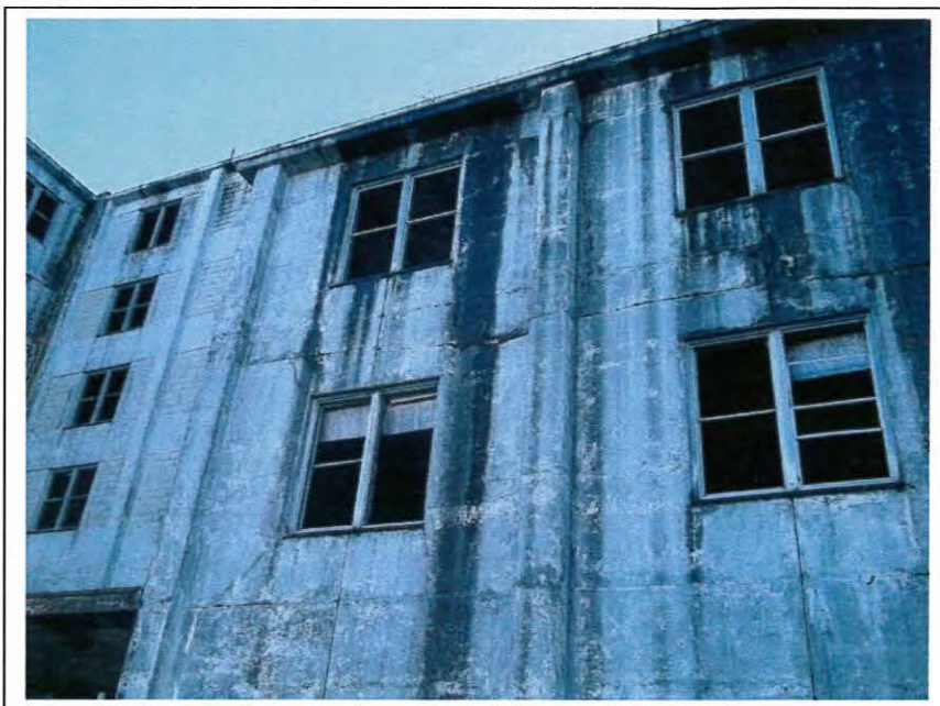
Photo H-39: Many exterior cracks appeared to form at individual floor levels; looking southeast. (October 22, 2014)
