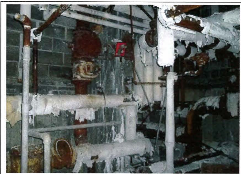
Photo H-14: Pressure reducing system and condensate return lines in the basement mechanical room. Note the white piping insulation is suspected of containing asbestos. (October 22, 2014)
