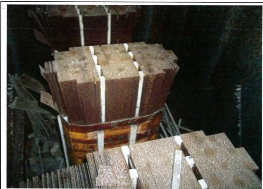
Photo H-10: Representative transformer plates in the Section A electrical distribution room. The transformer plates are suspected of containing asbestos. (October 22, 2014)
