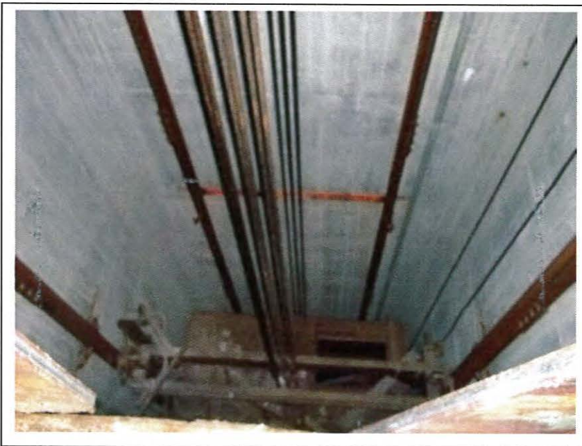
Photo H-26: Third floor elevator shaft without safety barricade or gate. (September 8, 2014)
