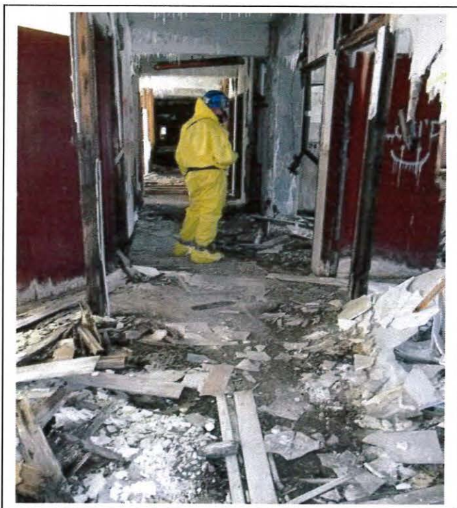
Photo H-25: Representative third floor hallway. Wallboard and ceiling tiles are suspected of containing asbestos. (September 8, 2014)
