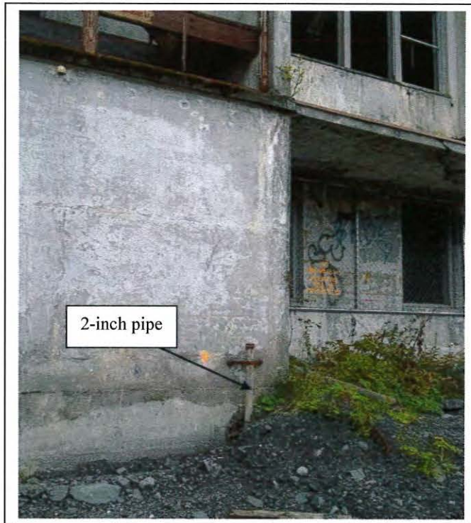
Photo H-31: Two-inch pipe observed near the northwest corner of Section C; looking southeast. Note that based on the size, location, and construction of the pipe, the pipe may be a vent pipe associated with an undocumented UST. (September 8, 2014)
