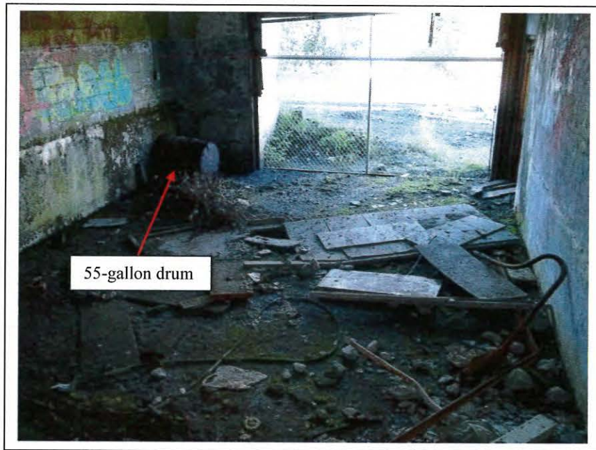
Photo H-21: One empty 55-gallon drum was observed in the ground floor unit of Section G. (October 22, 2014)
