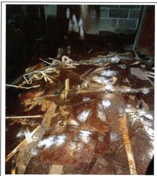
Photo H-11: Most transformer plates have been disassembled and discarded on the floor. Note the white spots on the transformer plates are minerals deposits that have dripped from overhead stalactites. (October 22, 2014)
