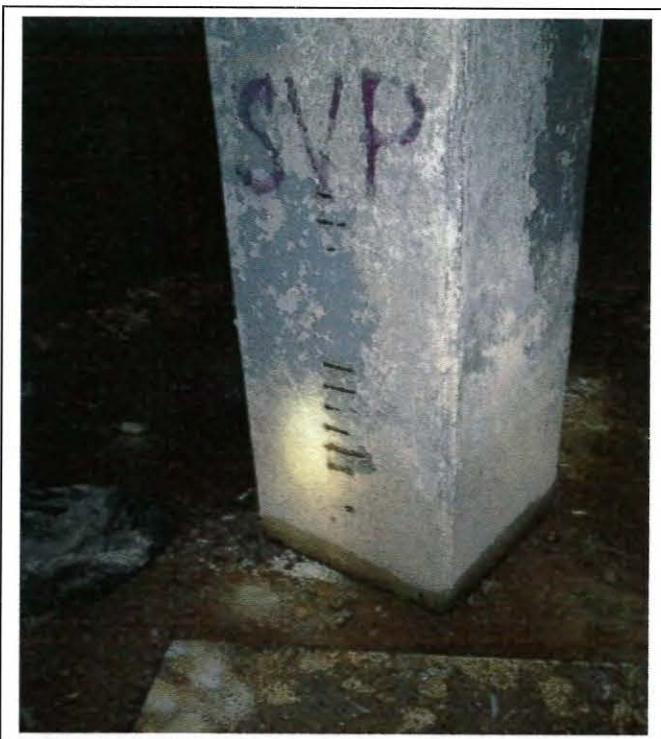
Photo H-23: Representative ground-floor structural column. Note that the concrete has spalled exposing the rebar. (October 22, 2014)
