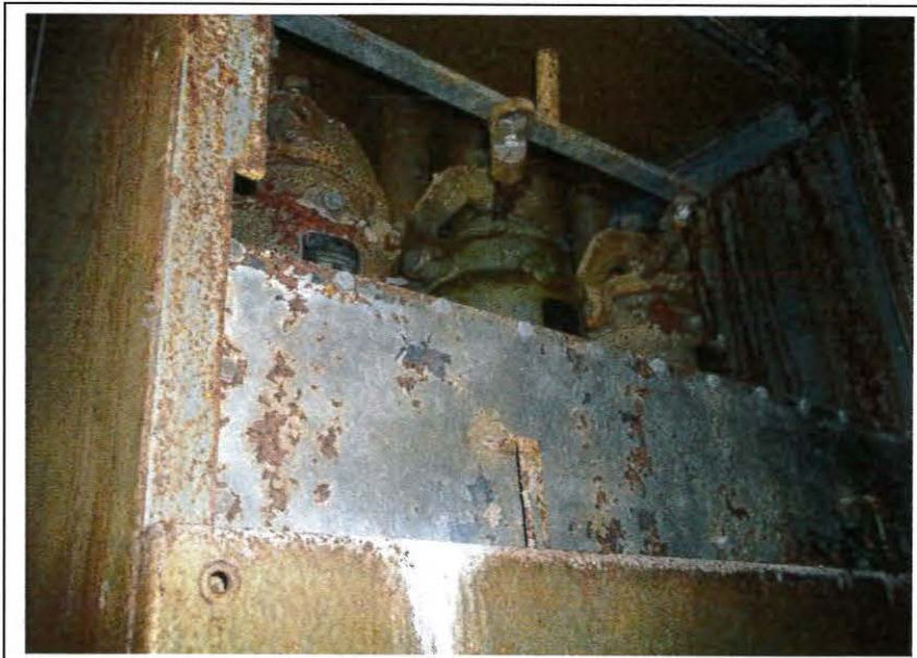
Photo H-18: It is presumed that the oil-filled switches remain intact behind the gray panel; electrical distribution room in Section E of the basement. (October 22, 2014)
