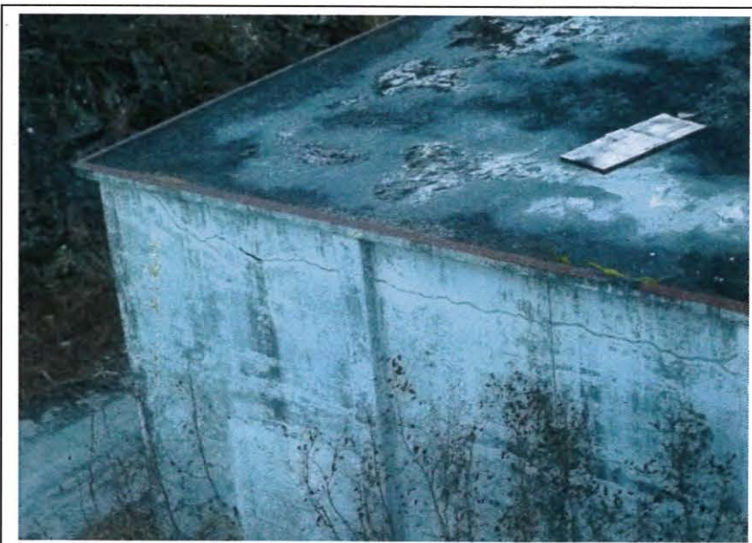
Photo H-38: Exterior crack observed in Section B; looking south from fourth floor Section A. (October 22, 2014)
