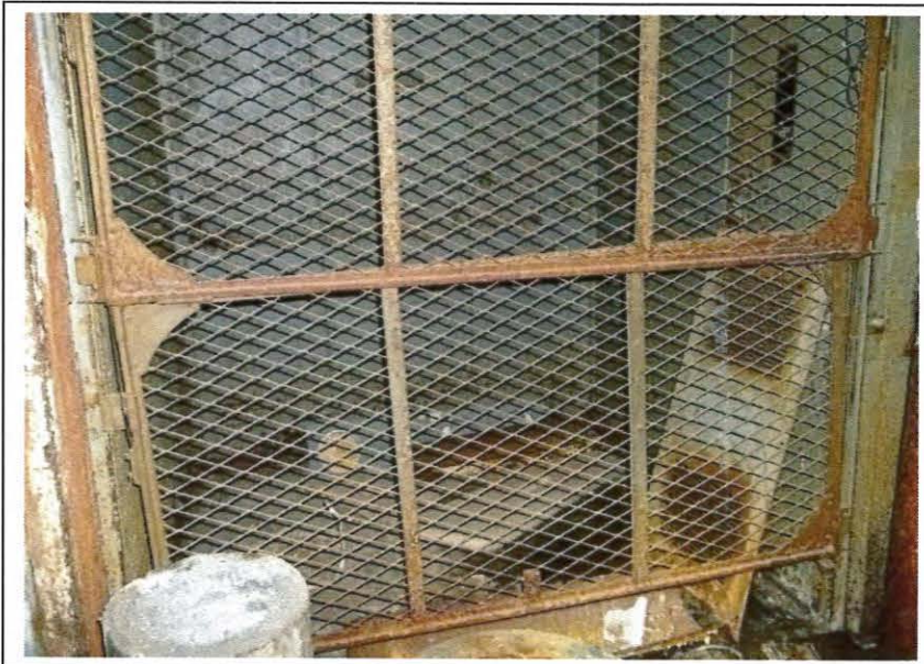
Photo H-2: Representative elevator. Note not all elevators had protective doors blocking the elevator shaft. (September 8, 2014)
