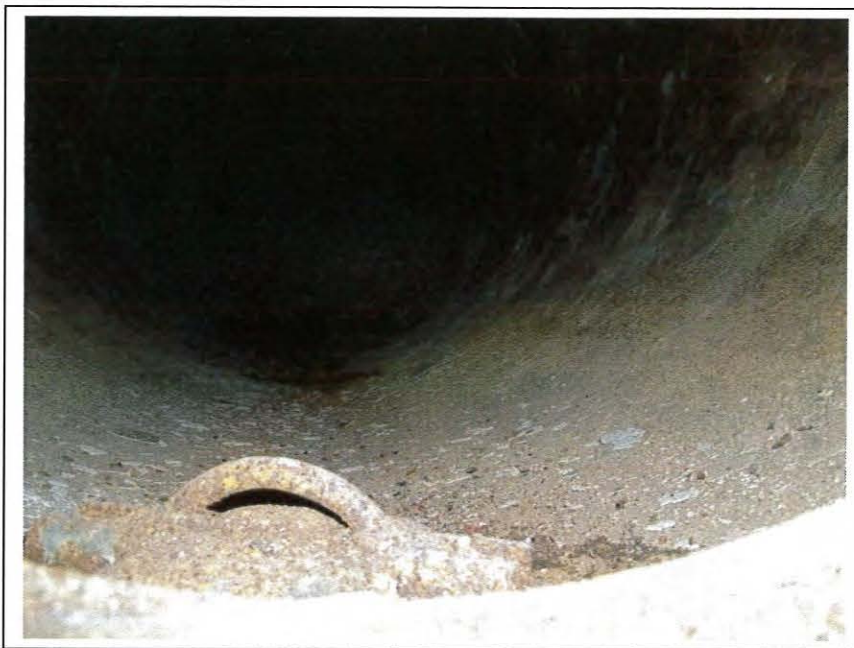
Photo H-13: Each of the two approximately 5,000-gallon tanks in the basement mechanical room are empty. It is presumed that the tanks were formerly used as hot water tanks. (October 22, 2014)
