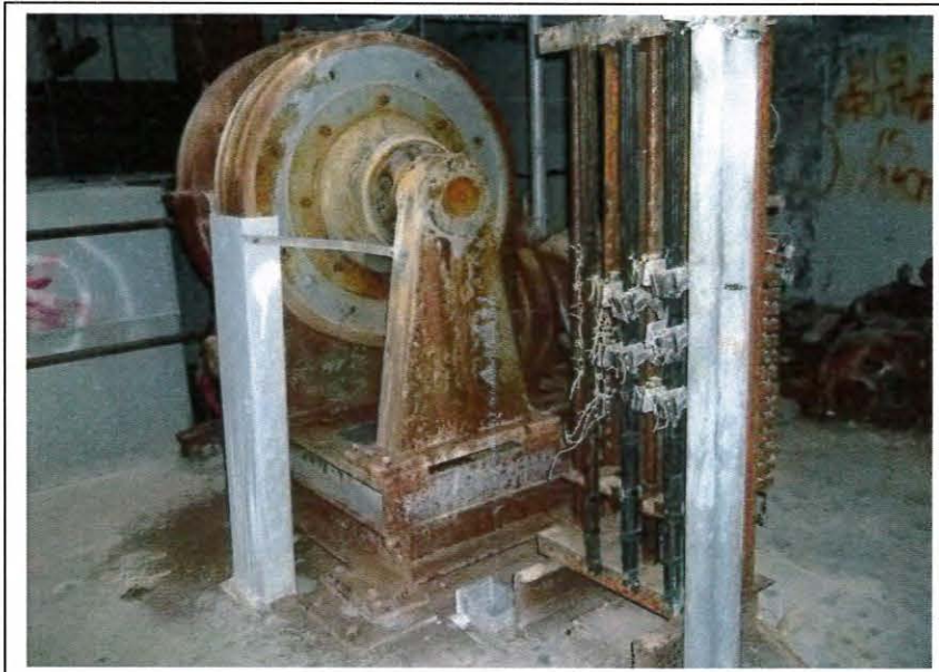
Photo H-28: Penthouse elevator platform. (October 22, 2014)
