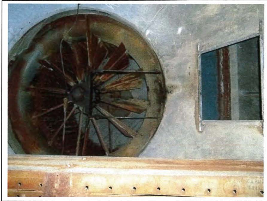
Photo H-27: Penthouse fan room. (October 22, 2014)
