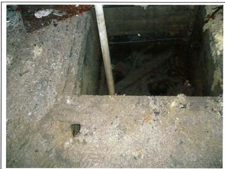
Photo H-15: The mechanical room sump contained standing water during each of our 2014 site visits. Note the floor is covered by a presumed asbestos slurry. (September 8, 2014)
