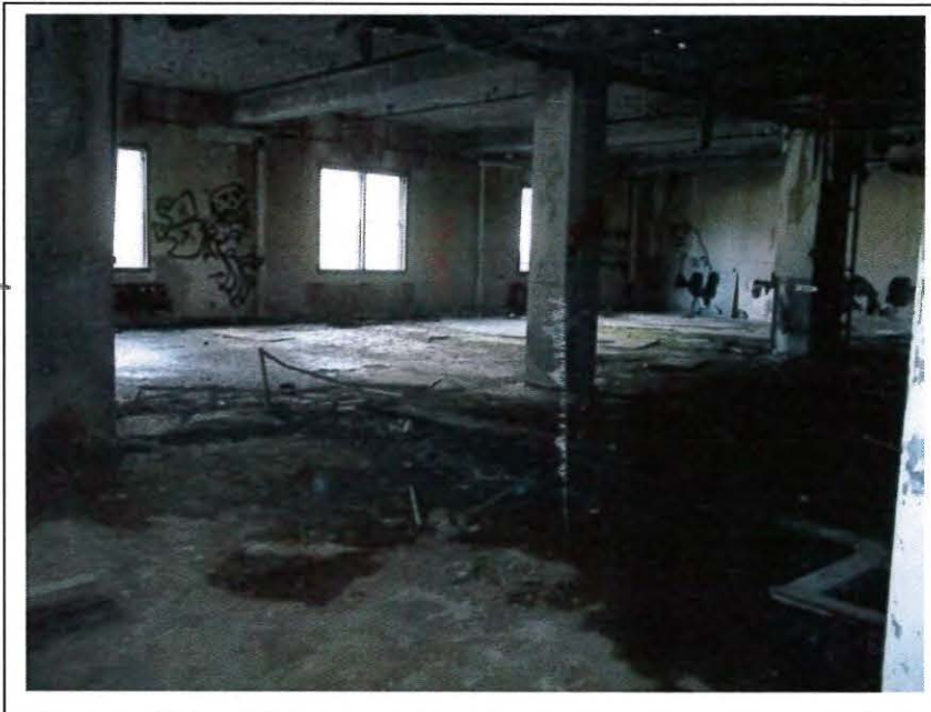
Photo H-4: Former owners and/or vandals have removed most valuables from the structure. In the photo above, the floor and ceiling tiles have been removed. (September 8, 2014)
