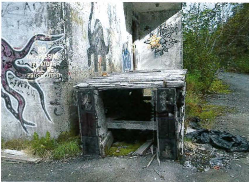
Photo H-36: Potentially creosote-treated railroad ties and litter observed near the southeast corner of the Buckner Building; looking northeast. (September 8, 2014)
