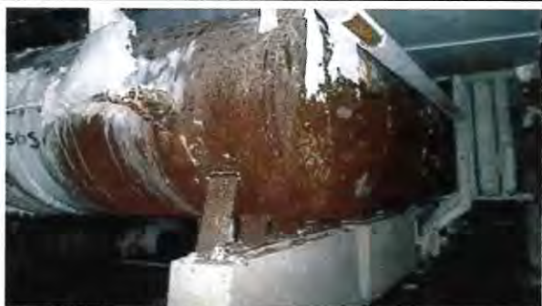
Photo 3: Two hot water tanks observed in the basement. Note the white insulation on the pipes likely contains asbestos. October 22, 2014.
