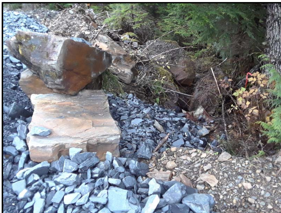
Photo 7: Looking east at the discharge endpoint of the French Drain system and sampling location MFD-01.
