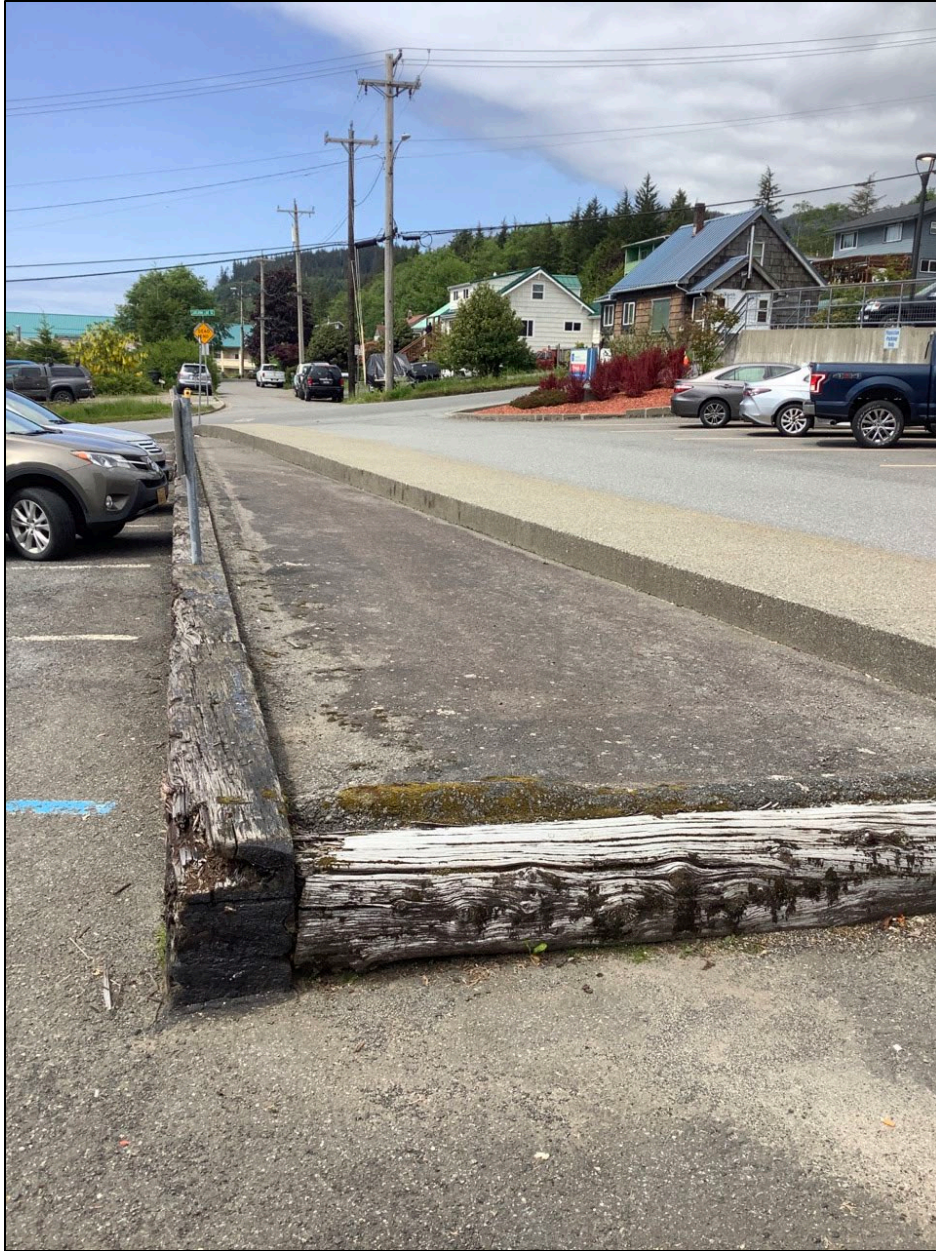
Figure 19. An unused paved area at 130 Carlanna Lake Rd. that could be converted to an infiltration basin or bioswale and capture and treat stormwater runoff from the upper parking lot and/or part of the lower lot.
