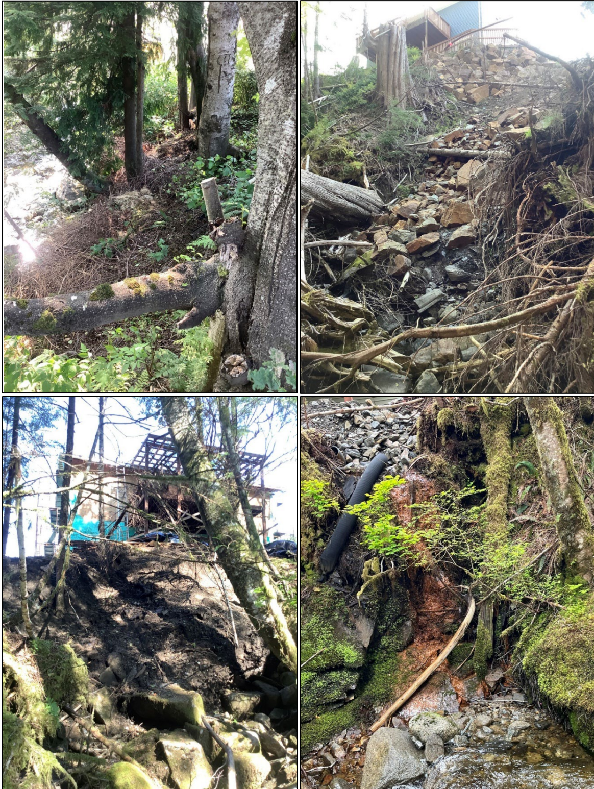
Figure 14. Damaged vegetation and erosion along Hoadley Creek. Top left: yard debris choking native vegetation. Top right: large rock and debris pushed over the terrace edge. Bottom left, Damaged vegetation and erosion below new construction. Bottom right: a displaced sediment filter sock and sediment-laden runoff below new construction.
