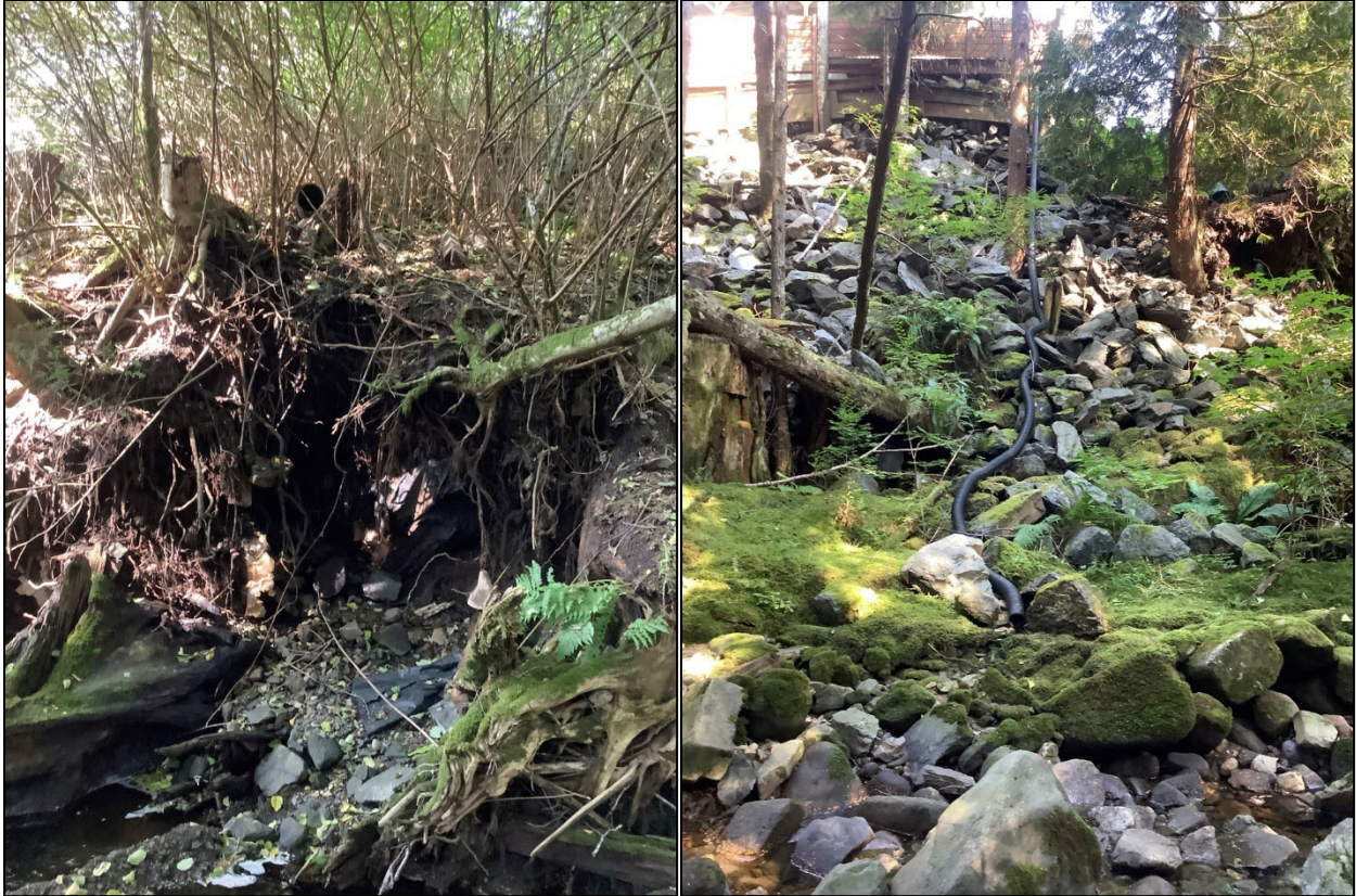
Figure 15. Local drains empty onto bare soil (left) or right next to the creek (right).
